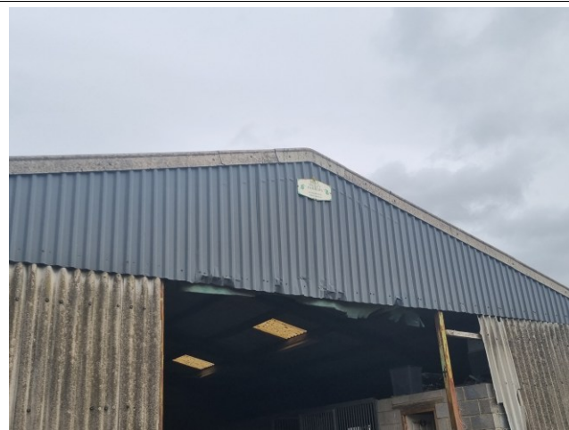
Photograph 7. Permanently open access to the building.
