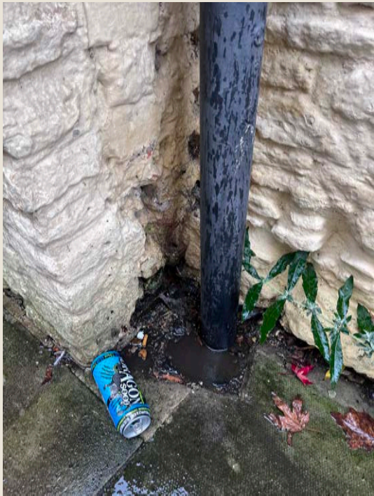
Figure 9: Southwest corner downpipe (RWP1) and hard paving around blocked gully
