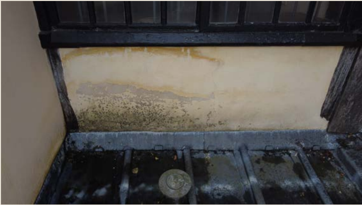
Figure 11: Water damage to wall above single storey metal roof, North elevation
