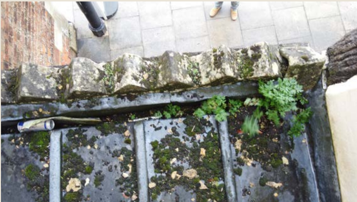
Figure 12: Metal roof with undersized parapet gutter (G7), significant vegetation and moss causing blockages. Damp and damaged dog-toothed stone parapet wall.
