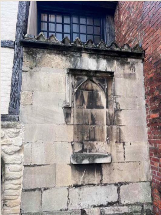
Figure 10: North elevation, damaged stone work to dog-toothed parapet and blank niche with missing right-hand stop
