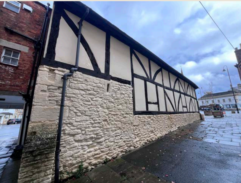
Figure 7: South elevation. Algae staining and rising damp to stone plinth. Southwest downpipe (RWP1) with multiple defective junctions and blocked gully
