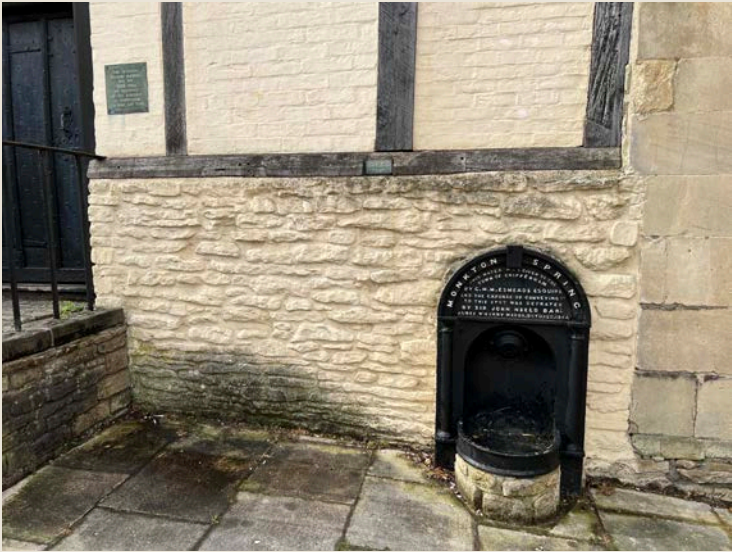
Figure 13: North elevation, significant damp due to lead valley discharging onto paving, with no rainwater runoff, and splashing back onto stone plinth
