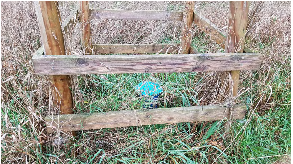
Plate 8: Photograph of existing borehole monitoring installations within eastern section of site.
