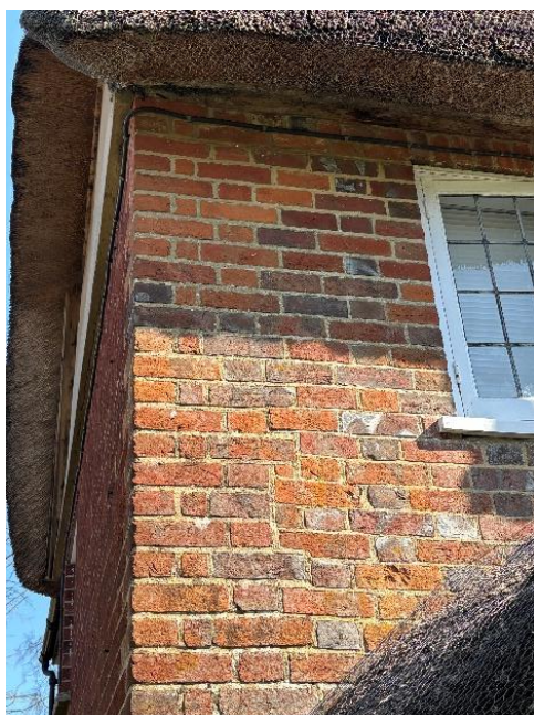
Fig.3 South-west corner showing discontinuity in brickwork due to the rebuilding of the north-east gable wall
