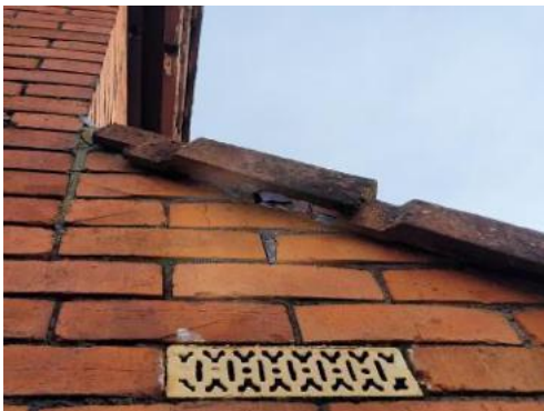
Photo 9: Gap between roof tile and wall of WC building.
