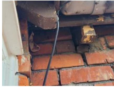
Photo 4: Loose brickwork around exposed rafter tail.
