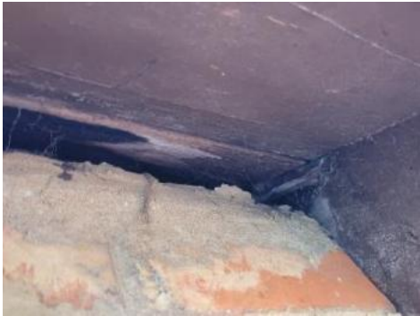
Photo 5: Gap between the wall top and roof.
