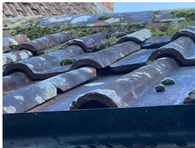
Image 10: Crevices beneath tiles of eastern link roof.
