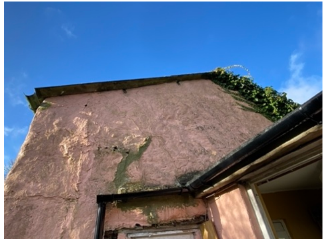
Image 2: View of eastern gable, with crevices at purlins.
