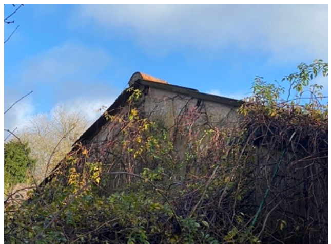
Image 6: Western gable end with crevices by purlins.
