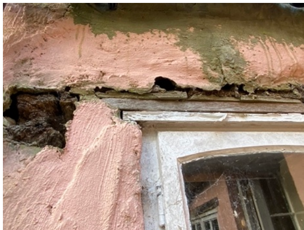
Image 8: Crevices above window on eastern gable.
