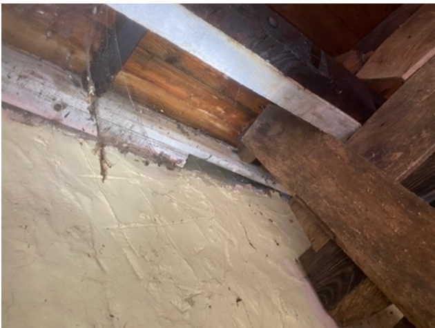
Image 15: Crevice where the southern lean-to roof meets the garage wall.
