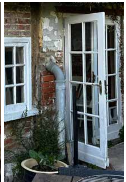
Drainage pipe to be removed and brickwork made good
