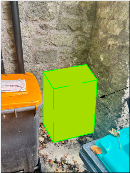
View "A" Heat main entry point
