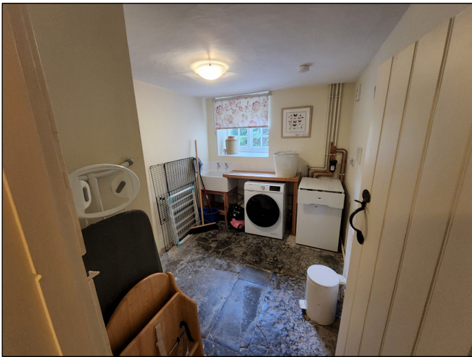
View "A". The Utility Room and Boiler
