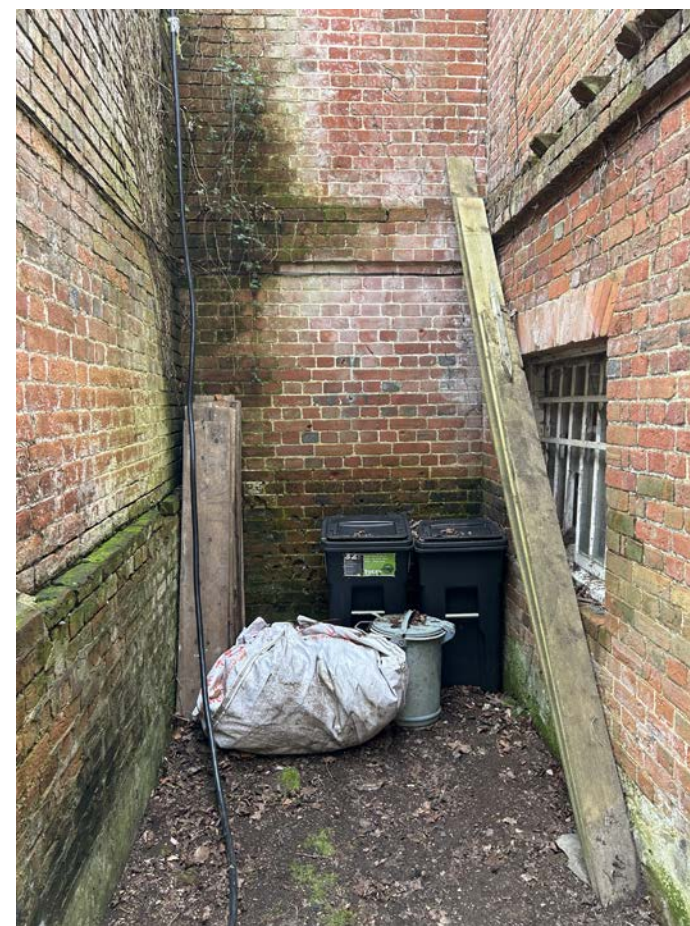
Figure 31. Unsatisfactory area created by the arrangement of the garden wall with the Coach House
