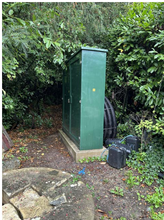
Figure 38. Electrical feeder post
