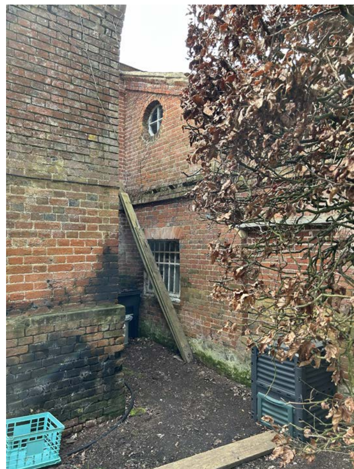
Figure 30. Unsatisfactory wall arrangement with the Coach House and north wall of the walled garden
