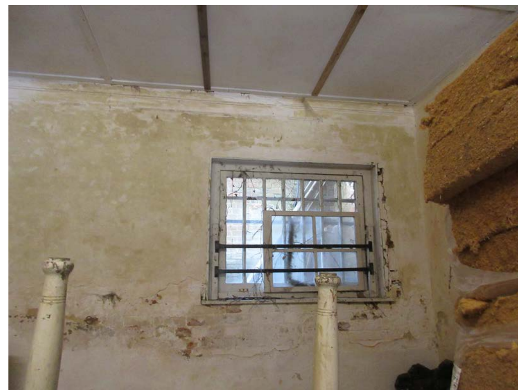
Figure 33. Dampness inside Coach House
