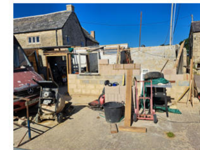
Standalone Farm Storage (4)
