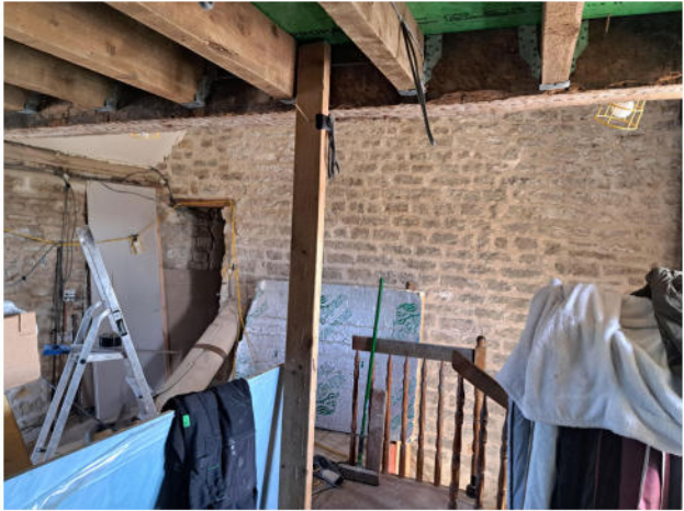
R Back room with top of spiral stair. Exposed wiring
