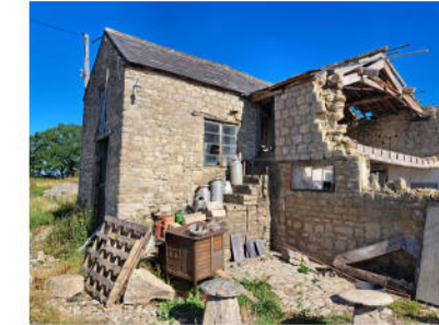
Derelict Dairy Barn (8)
