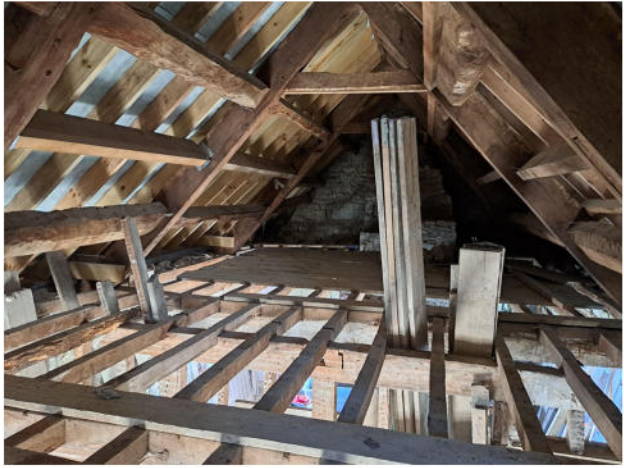
D Main loft with missing floor
