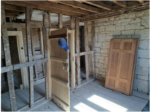
H Exposed wall studs and door DF02
