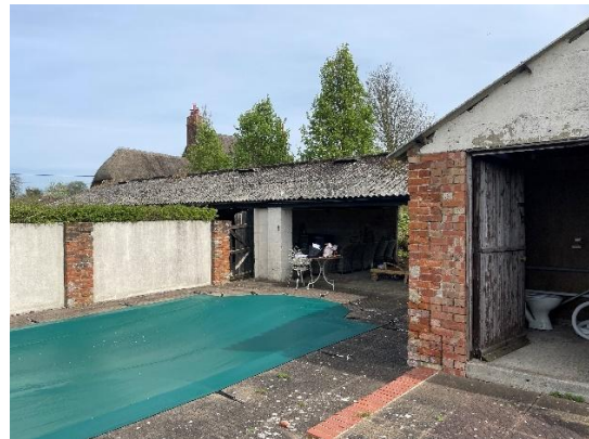
Fig 14 – View from poolside showing WC within storage barn, and garage outbuilding running north to south behind. Garden just visible beyond. Deteriorating concrete and brick patio paving visible.
