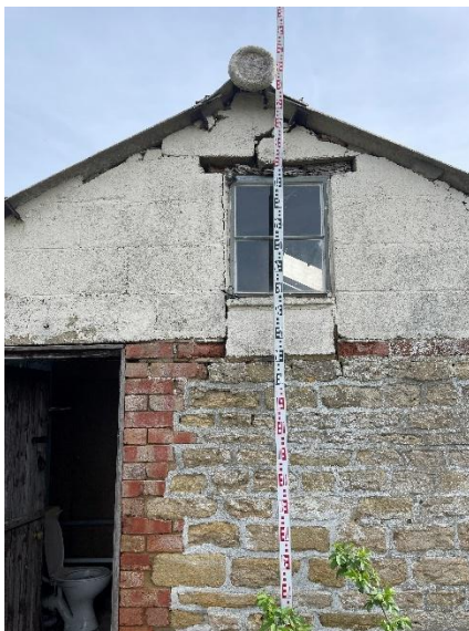
Fig 15 – View of west gable of storage barn with cracks visible over window and deteriorating lintel and masonry.
