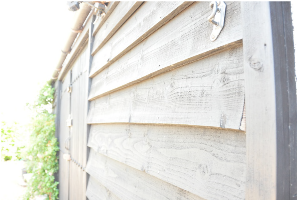
Plate 10 double nailed weather boarding on the long barn reduces access potential
