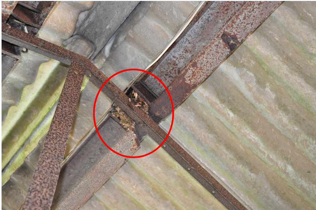
Plate 9 old bird nest in the roof of the long barn and open ridge with no beam
