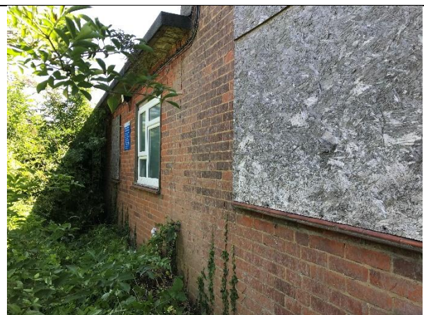
Photograph 18. B22, north side, boarded up windows with gaps behind
