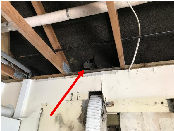
Photograph 13. B16, hole in roof felt corresponding with soffit access on east side
