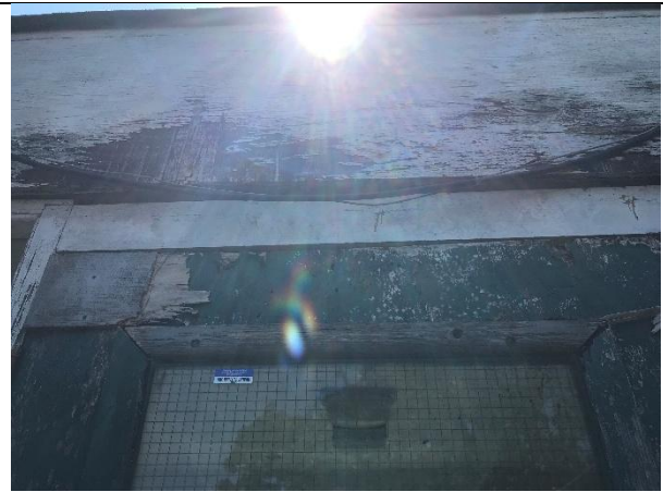
Photograph 16. B17, north side, gap in door frame
