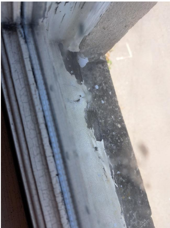
Example of sill rot in window C
