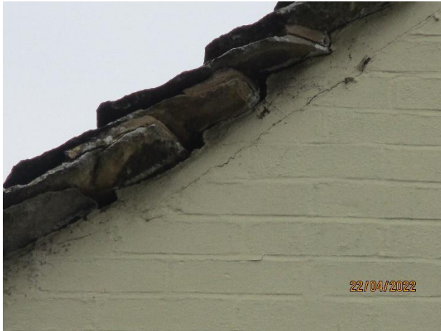
Photo 13: Gaps at the verges at the gable ends of the hotel.
