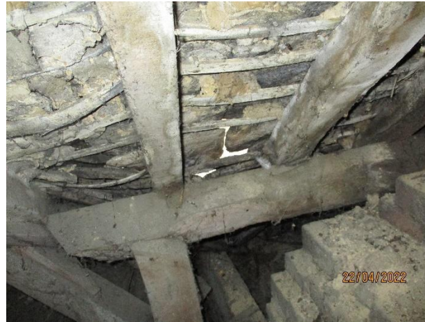
Photo 32: Area of no lining in 'Void 3'.
