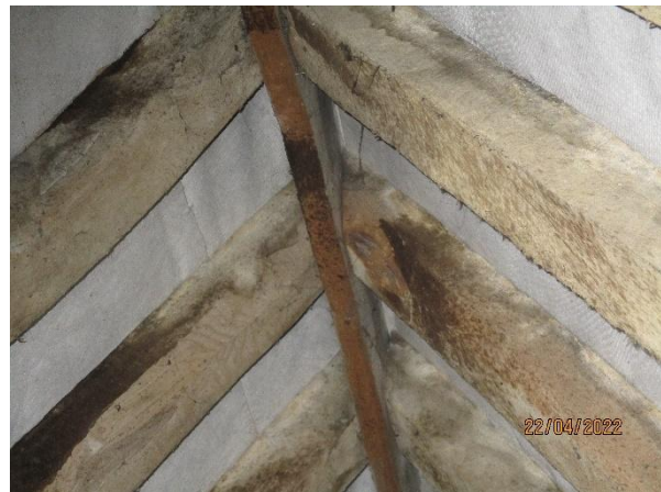
Photo 28: Staining at the ridge beam in 'Void 2'.
