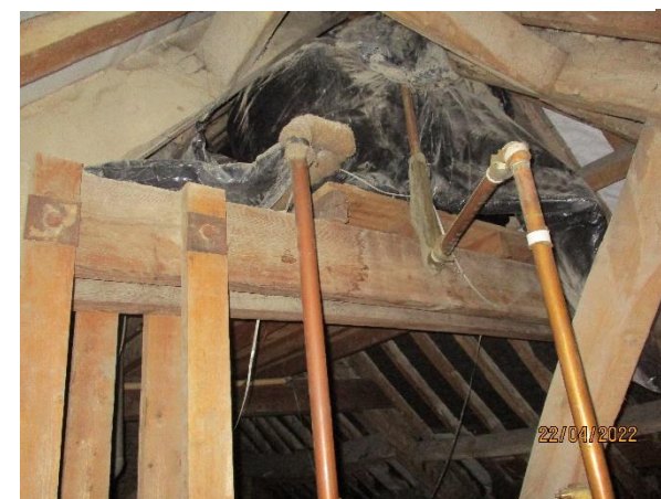
Photo 24: Water tank in 'Void 1' of the hotel.
