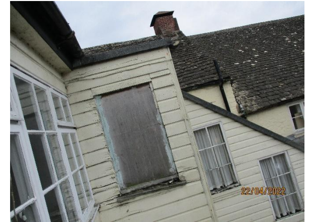
Photo 9: Wooden clad upper half of the hotel within the central courtyard and boarded up window.
