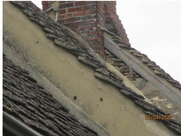
Photo 14: Gaps in the tiles at the verges of the gable ends on the western pitch.
