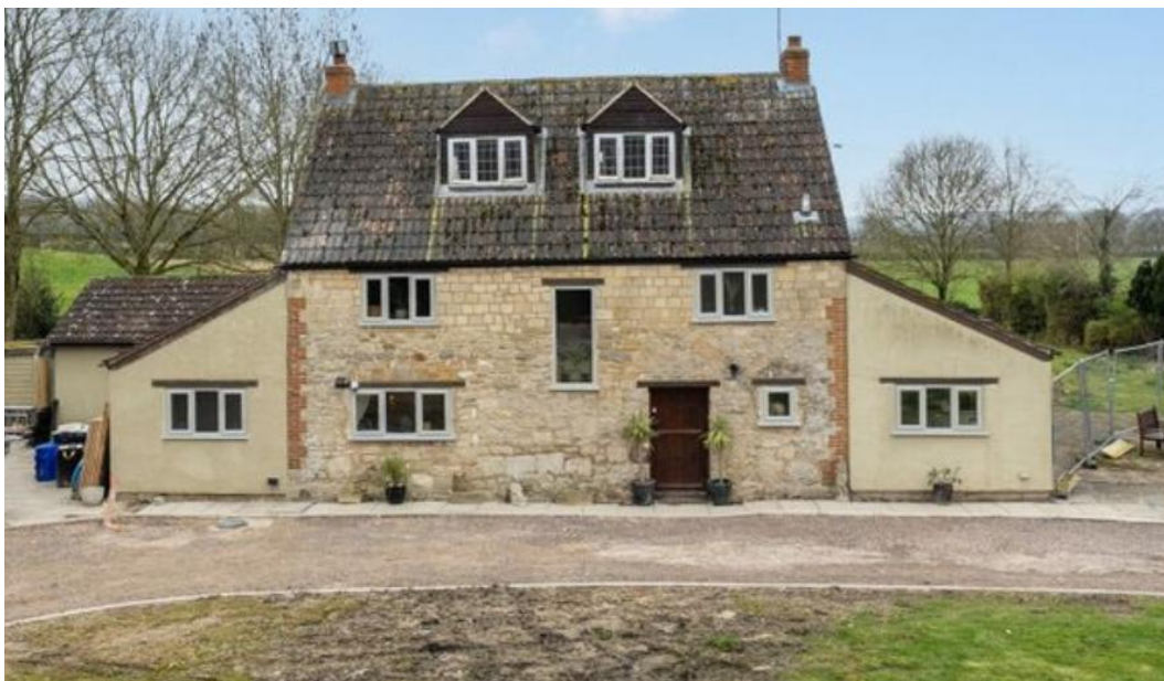
Recent image of front of property taken from sales brochure showing condition of stonework
