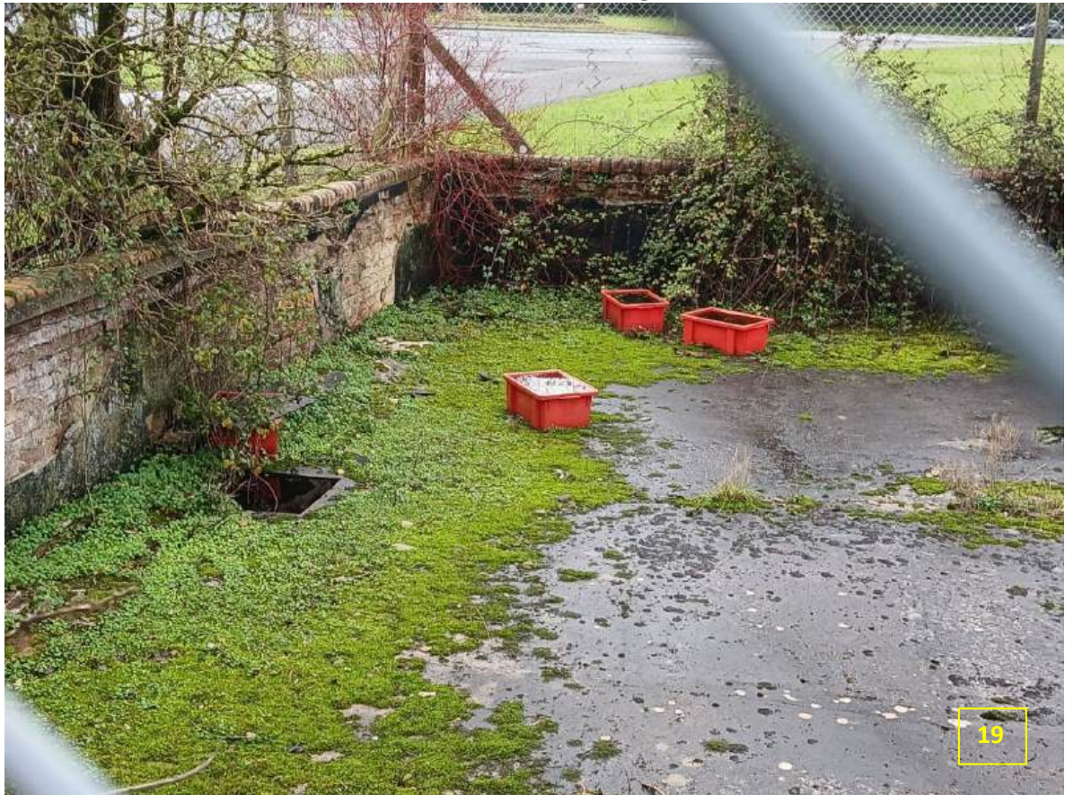
Water outlet/drain in storage basin
