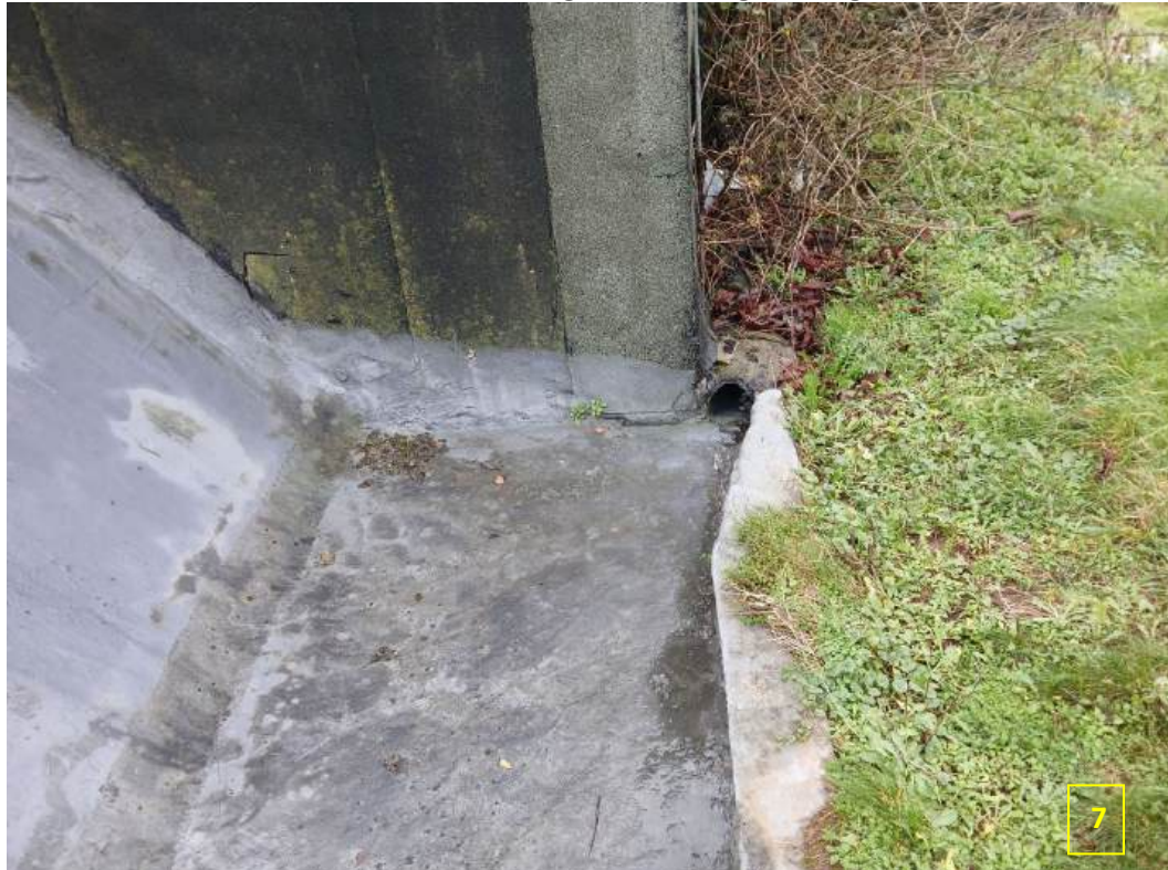
Water runoff and hangar 18 coating. (Facing W)
