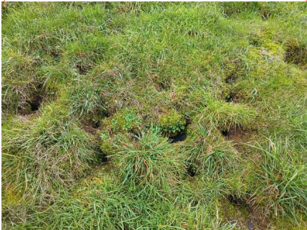
Several random holes in embankment
