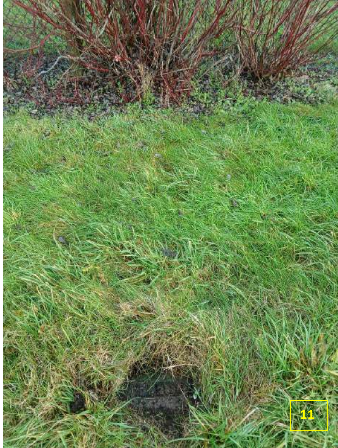
Overgrown electric warning brick parallel to fence line (Facing E)
