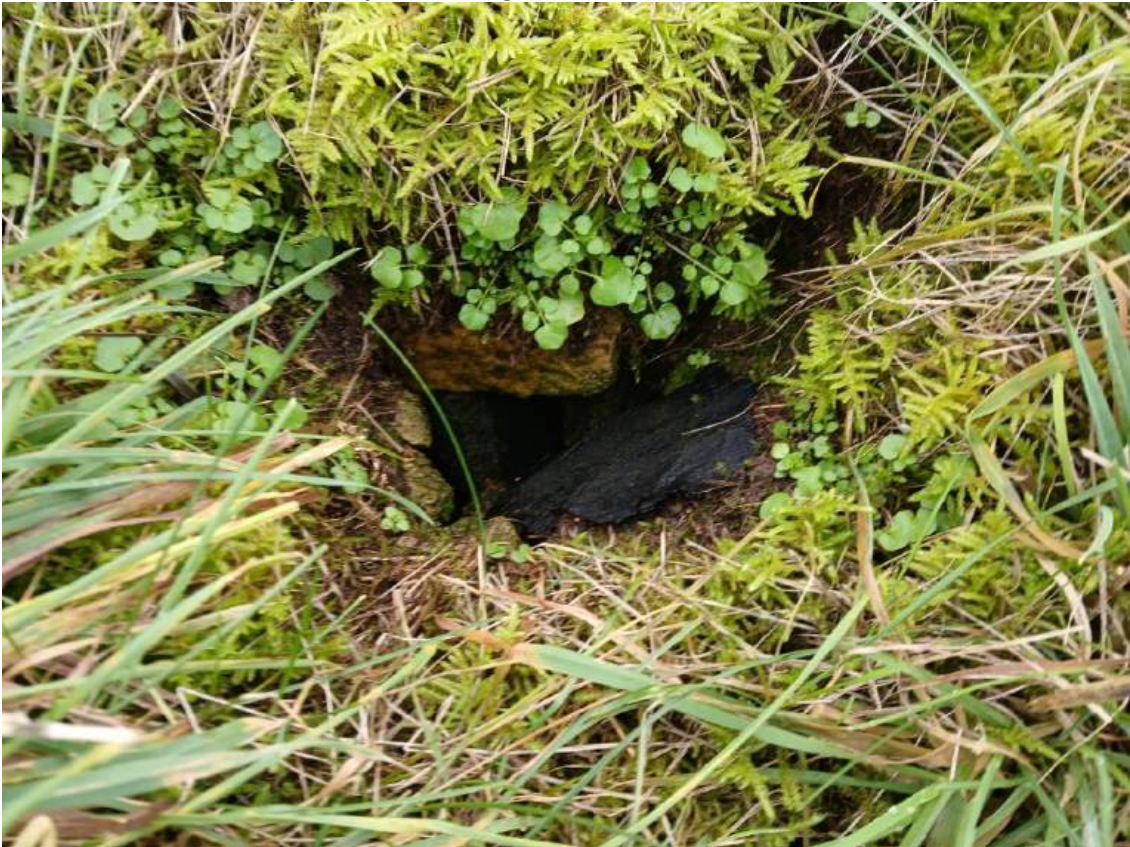
Possible locally collapsed underground structure. Black membrane pieces.
