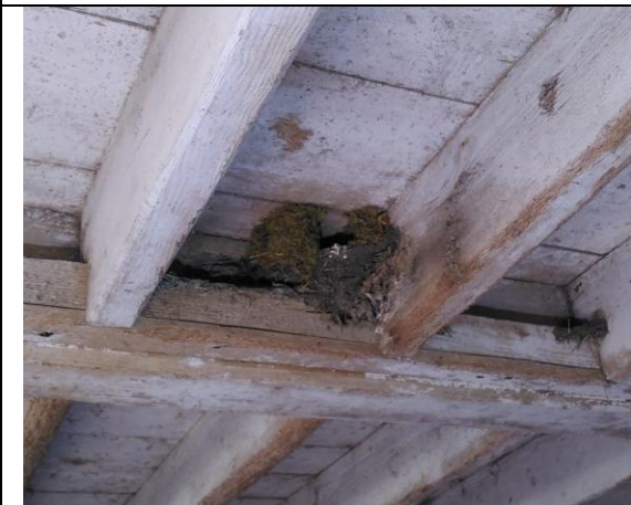
Fig 24. Bird nest fixed to the rafters. Photo taken 20 th April 2026.
