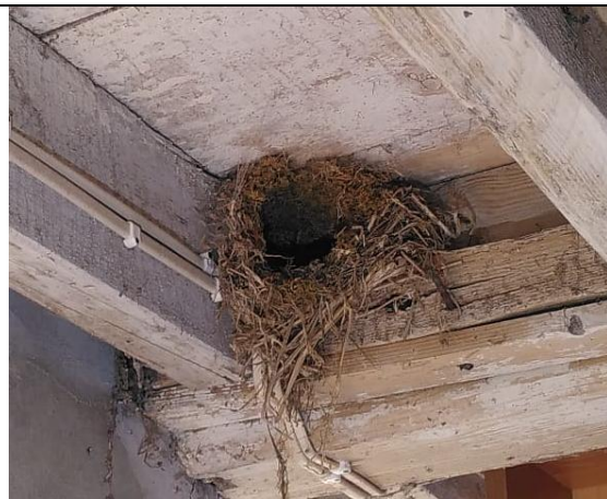
Fig 25. Bird nest fixed to the rafters. Photo taken 20 th April 2026.
