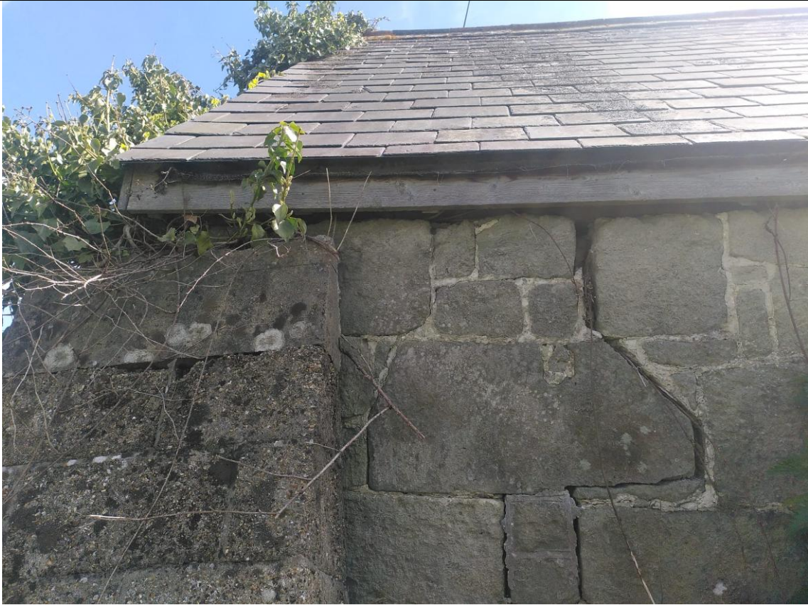
Fig 14. Western elevation: on the northern end several large cracks were present in the wall, providing potential roost features as well as access to the interior. Photo taken 20 th April 2026.
