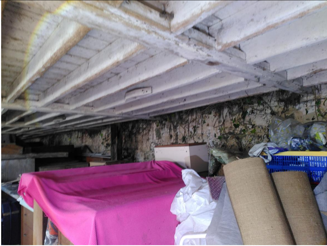
Fig 18. Ivy had grown through the eaves and into the room from the western elevation. Photo taken 20 th April 2026.
