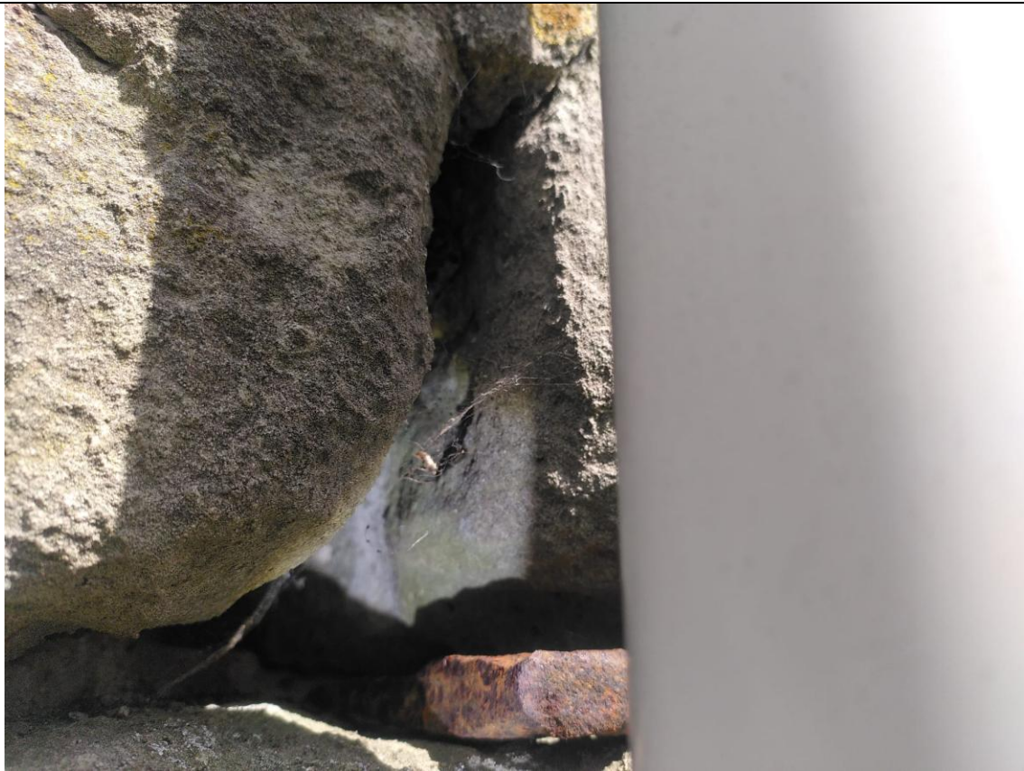
Fig 12. Southern elevation: a substantial cleft behind the downpipe. Photo taken 20 th April 2026.
