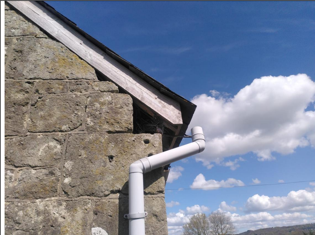
Fig 23. Southern elevation: many sticks were evident in the largest of the holes at the base of the gable end in the righthand corner. Photo taken 20 th April 2026.
