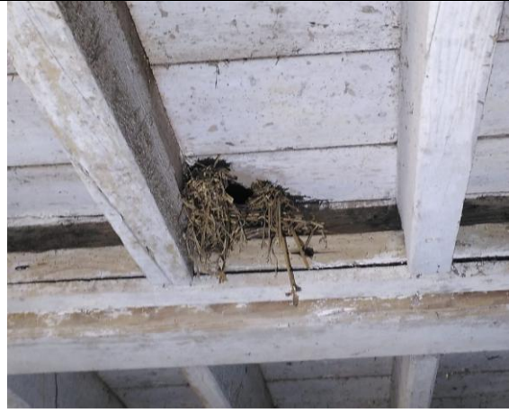
Fig 27. Bird nest fixed to the rafters. Photo taken 20th April 2026.
