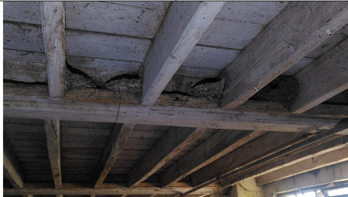
Fig 28. Bird nest fixed to the rafters. Photo taken 20th April 2026.
