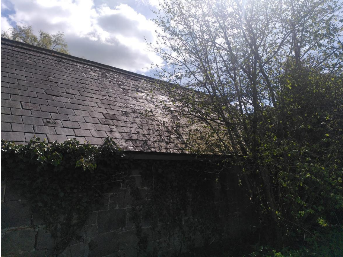
Fig 13. The western elevation: ivy encroaching on the walls up to the eaves in places. Photo taken 20 th April 2026.
