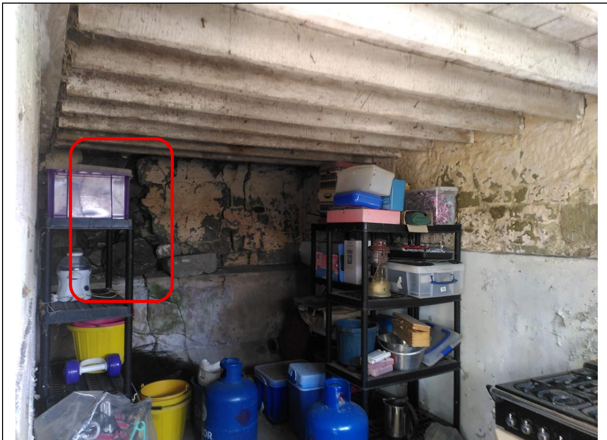
Fig 17. The block work has deteriorated over time and caused many crevices in the back (western) wall, especially toward the north end. Photo taken 20 th April 2026.
