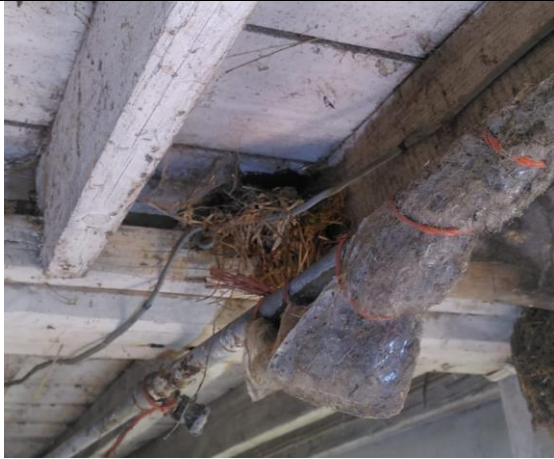
Fig 26. Bird nest fixed to the rafters. Photo taken 20th April 2026.
