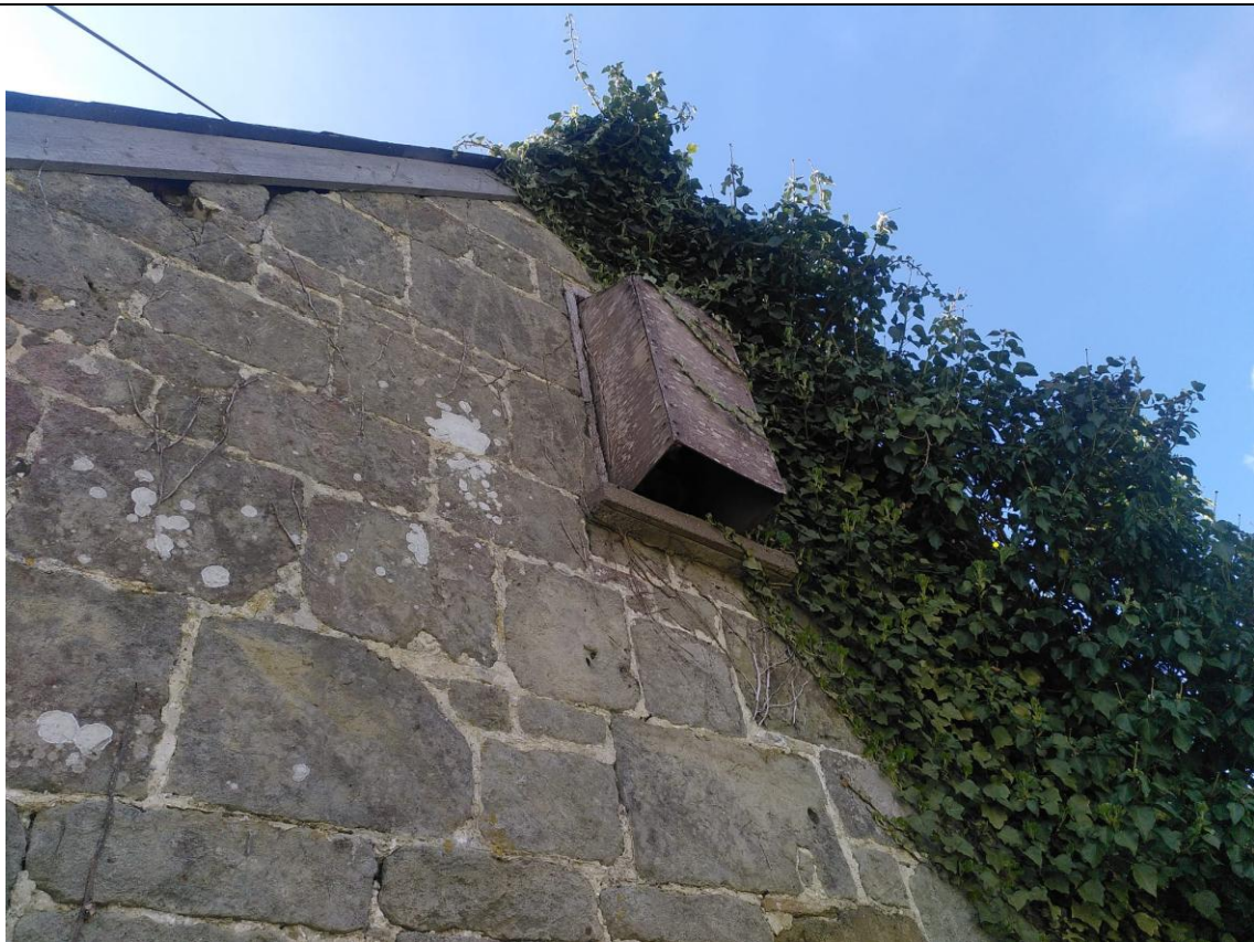
Fig 16. Northern elevation: the centre of the gable end had a box fixed over the window which was fully open at the base and loosely attached all around. Photo taken 20 th April 2026.
