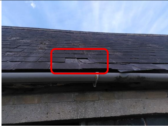
Fig 8. Eastern elevation: missing slate at the centre. Photo taken 20 th April 2026.
