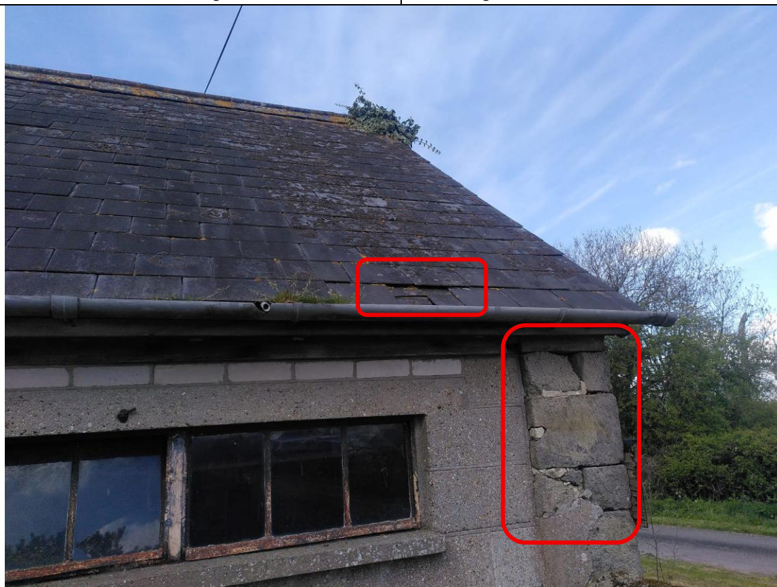
Fig 10. Eastern elevation: missing slate at the northern end of the eastern roof and the cracks on the northeastern corner. Photo taken 20 th April 2026.
