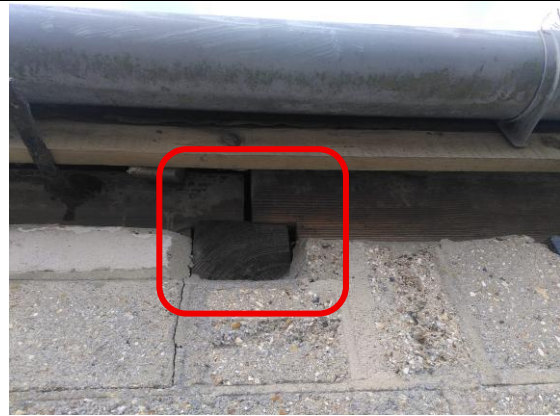
Fig 9. Eastern elevation: gap at joist. Photo taken 20 th April 2026.
