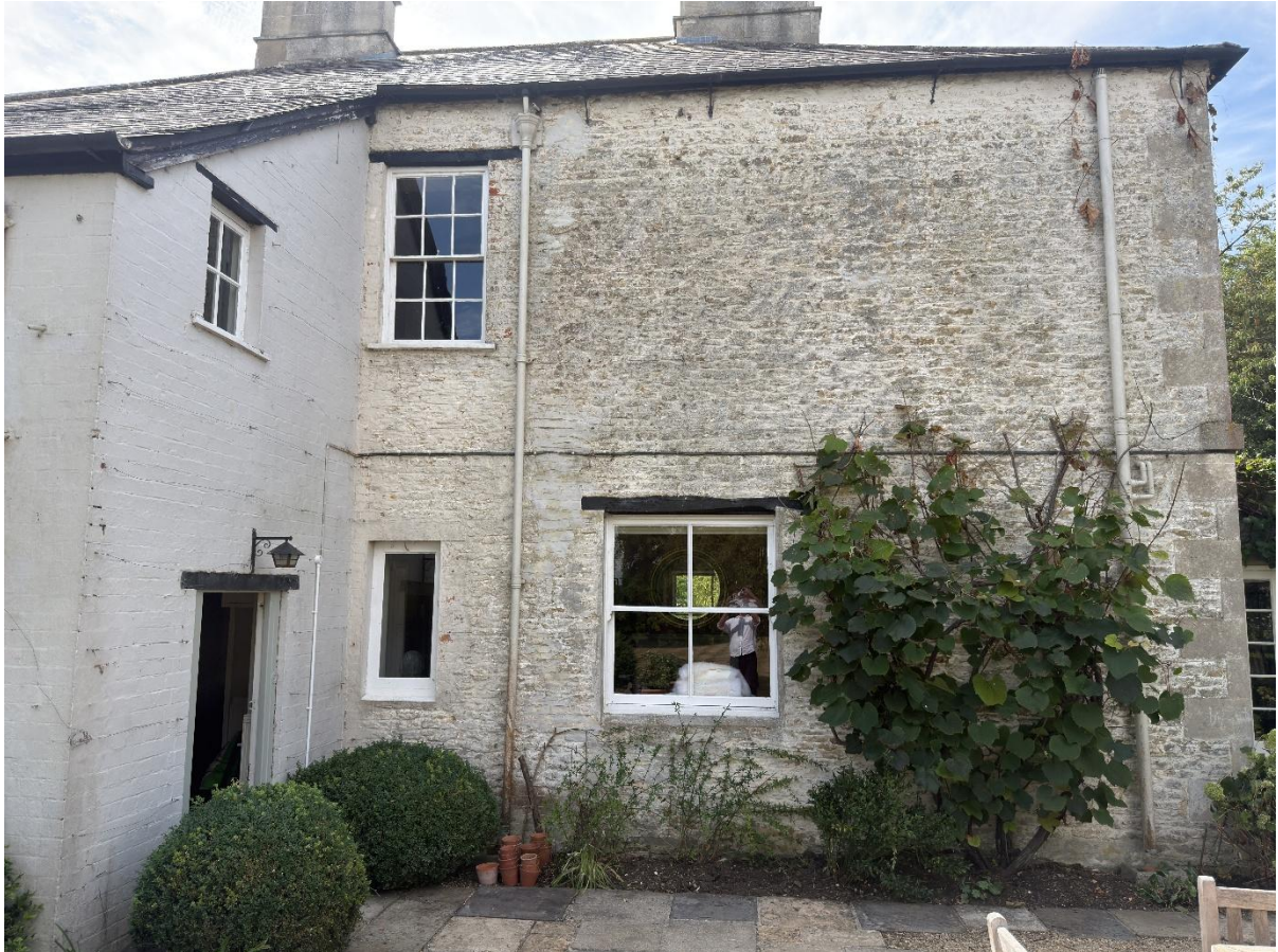
Figure 7. Elevation with poor cementitious render to be locally removed and replaced with lime render.
