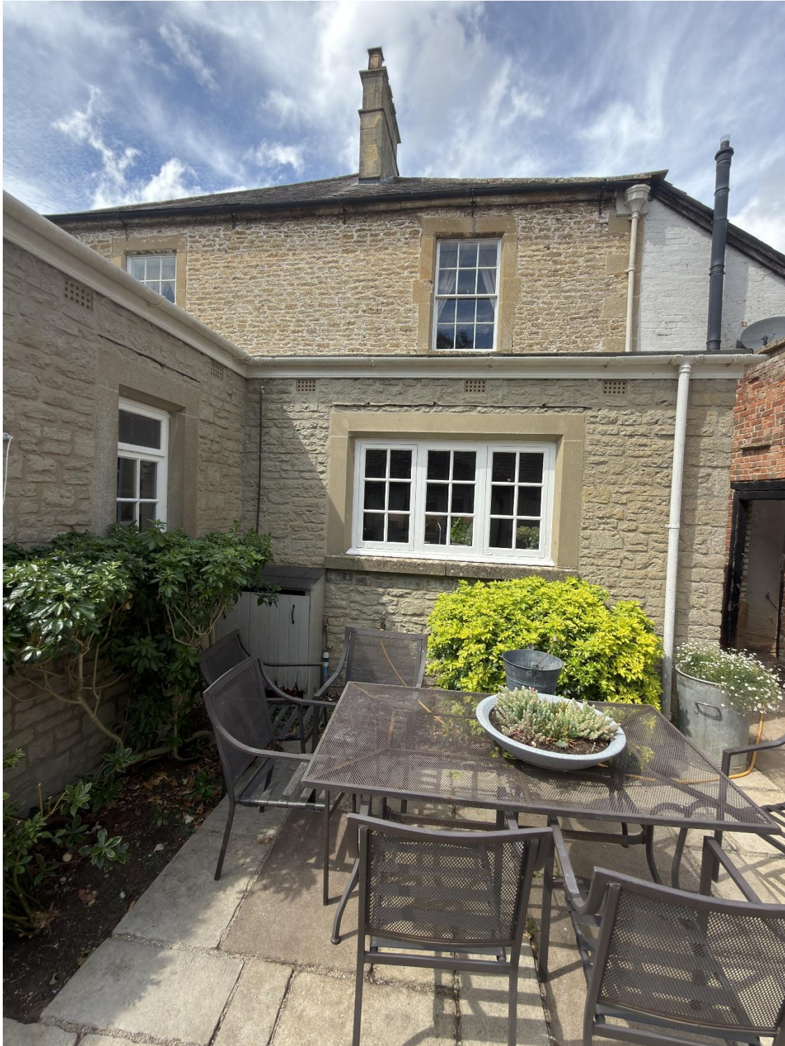
Figure 2. Existing condition of window sill to be lowered in proposal (area A)
