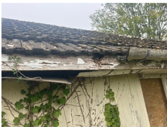
Photo 9: Damaged timber soffit.
