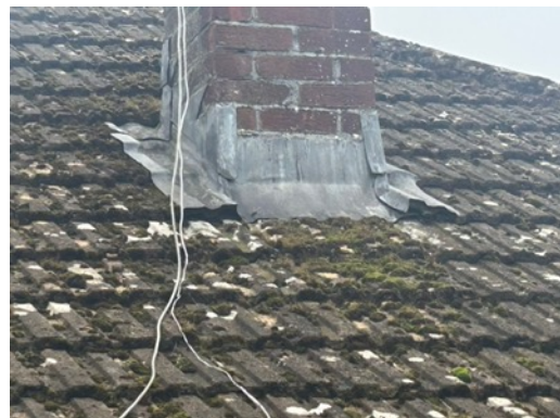
Photo 6: Gaps leading beneath lead flashing lining chimney base.
