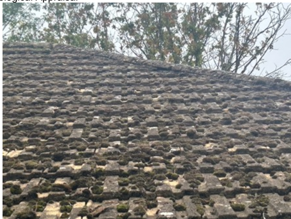
Photo 7: Concrete roof tiles, largely flush and tightly fitted, and with gap leading beneath failed bedding mortar.
