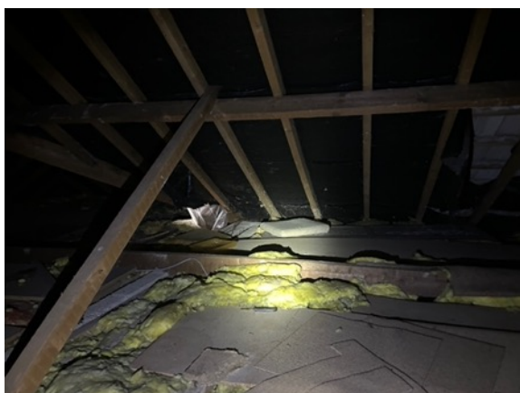
Photo 11: Internal view of loft void with light ingress at roof eaves.
