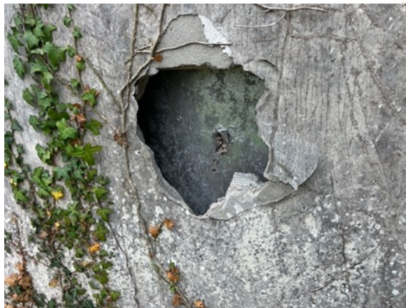
Photo 8: Damaged concrete render at eastern elevation.
