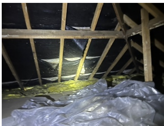
Photo 10: Internal view of loft void within torn and sagging felt.
