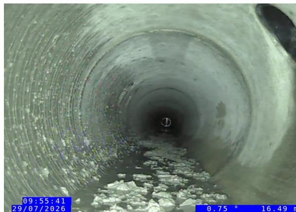
6, 00:03:23, 16.49 m Settled deposits, fine, 10% cross-sectional area loss
