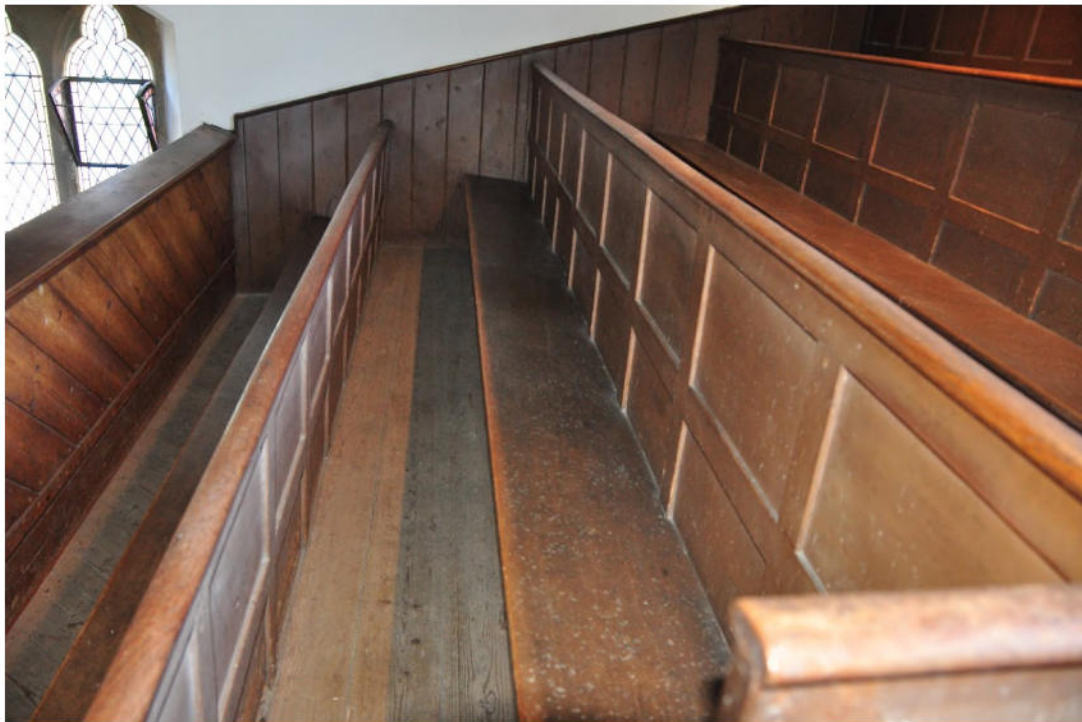
Plate 22 pitting on pews from bat urine splashing
