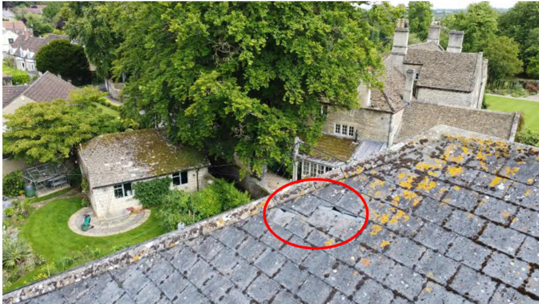
Plate 11 cracked roof tiles but no evidence of use by bats
