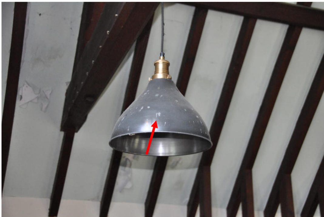
Plate 6 bat urine staining on interior lamp shade (white marking)
