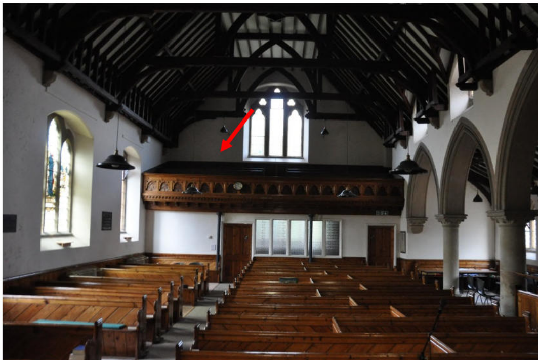
Plate 4 showing the balcony area which has evidence of scattered bat droppings
