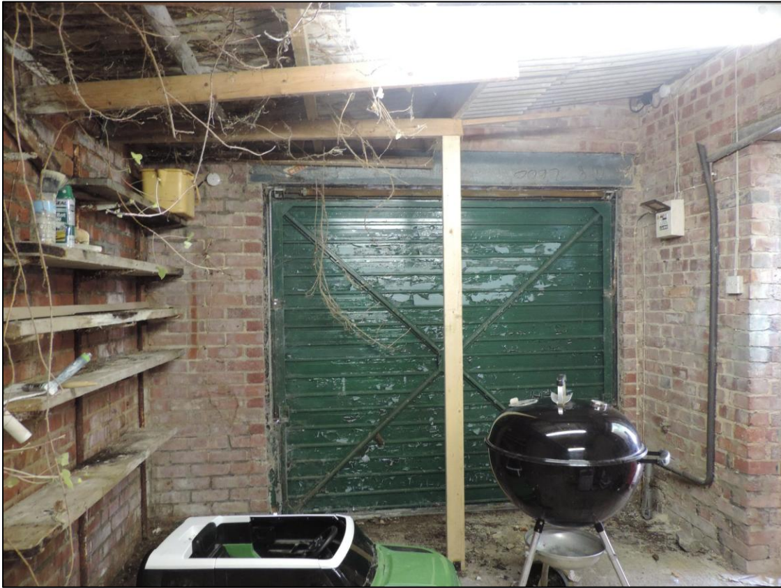
Photo 4 North-west facing view within garage towards door blocked by timber supporting roof.
