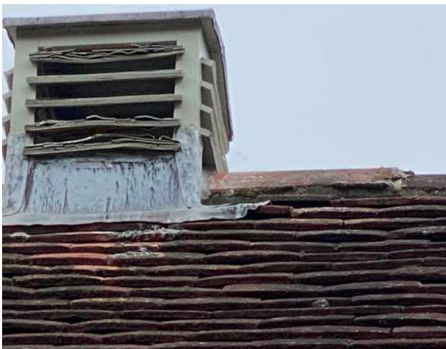
Image 11: Example of lifted tiles, gaps around the lead flashing around the vents at the ridge.
