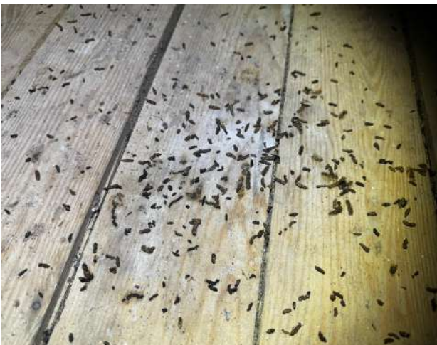
Image 5: Droppings in void A on update inspection June 2026
