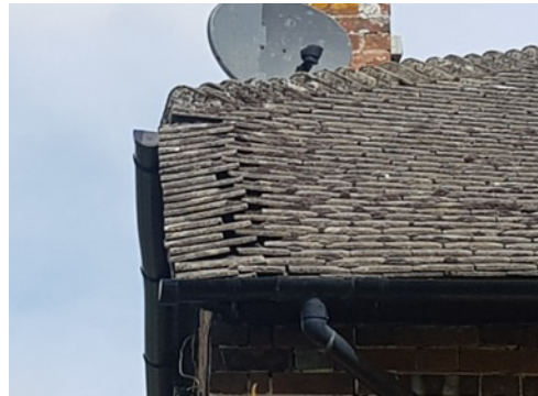
Photo 4: B1 - Gaps under tiles of southern roof aspect
