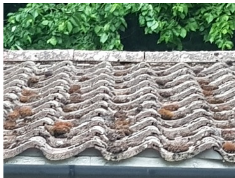
Photo 10: B2 - Single small gap leading beneath ridge tile.
