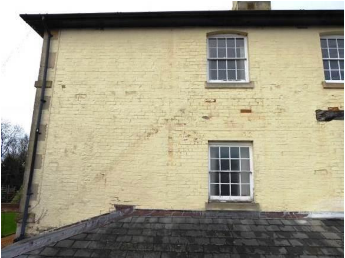
Fig 8.1.6: Scar of removed fire escape stairs and top landing
