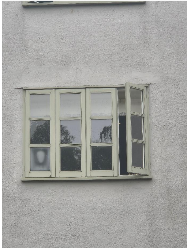
Existing first floor casement window (middle right). Note failed/blown pane at bottom left.
