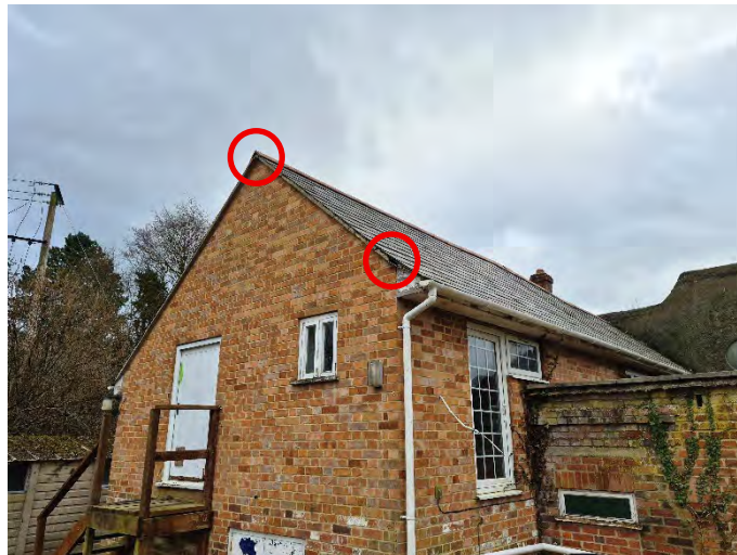
Figure 13: Gaps present under tiles
