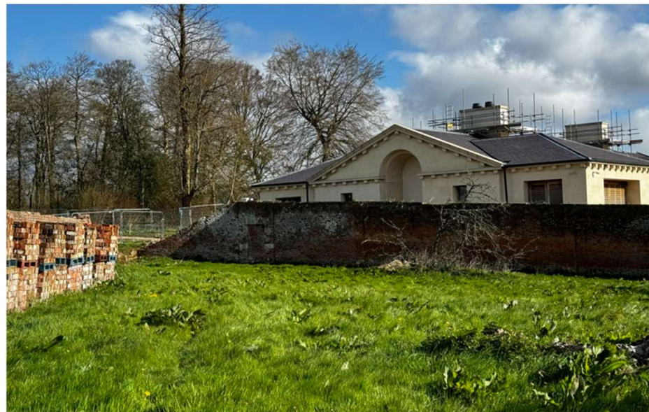
Figure 7 – View toward the Energy Centre
