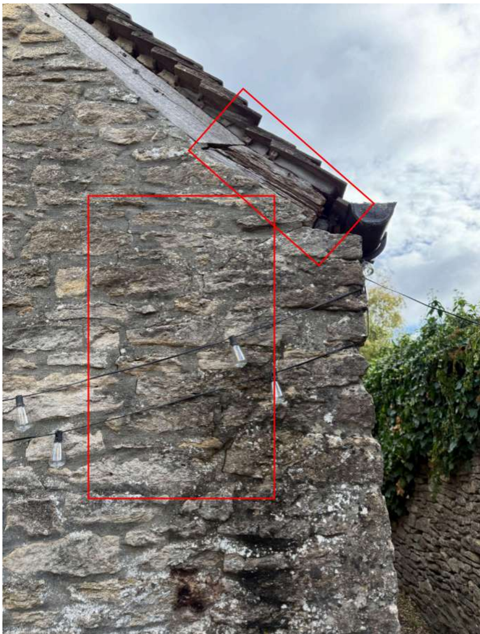
Picture 5 - Righthand side of gable wall damp stonework with hairline cracks and timber rot
