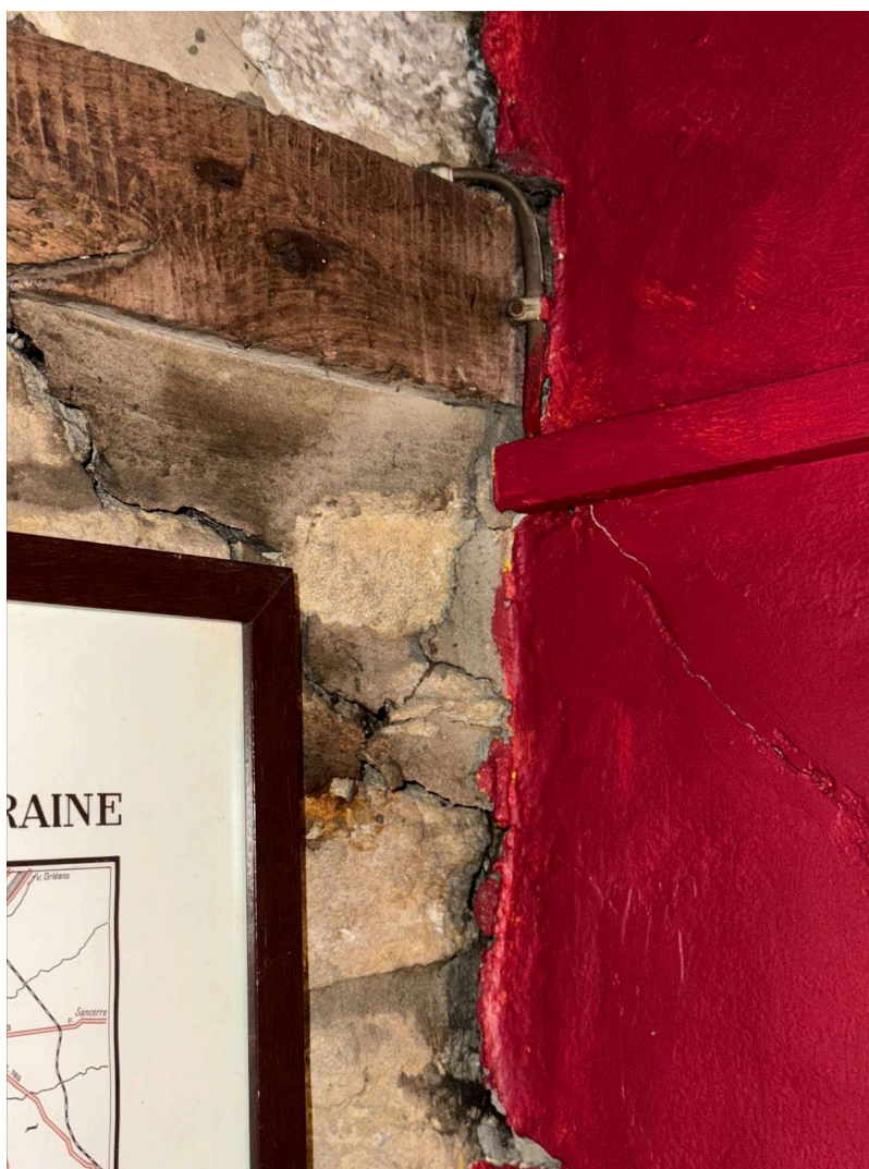
Picture 11 - Stepped crack below the righthand timber strap in the gable wall
