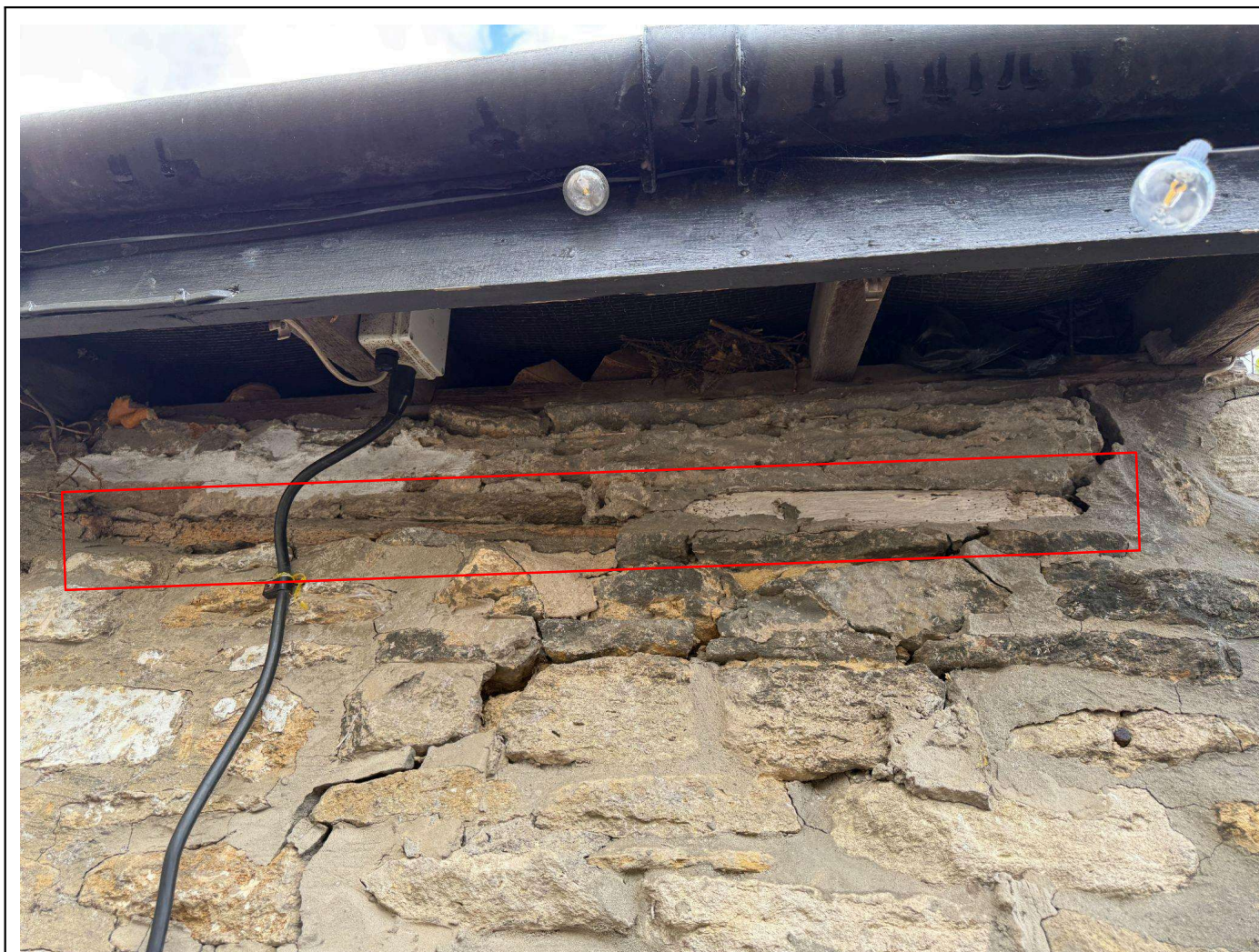
Picture 2 - Deteriorated stonework to the eaves level and exposed timber beam
