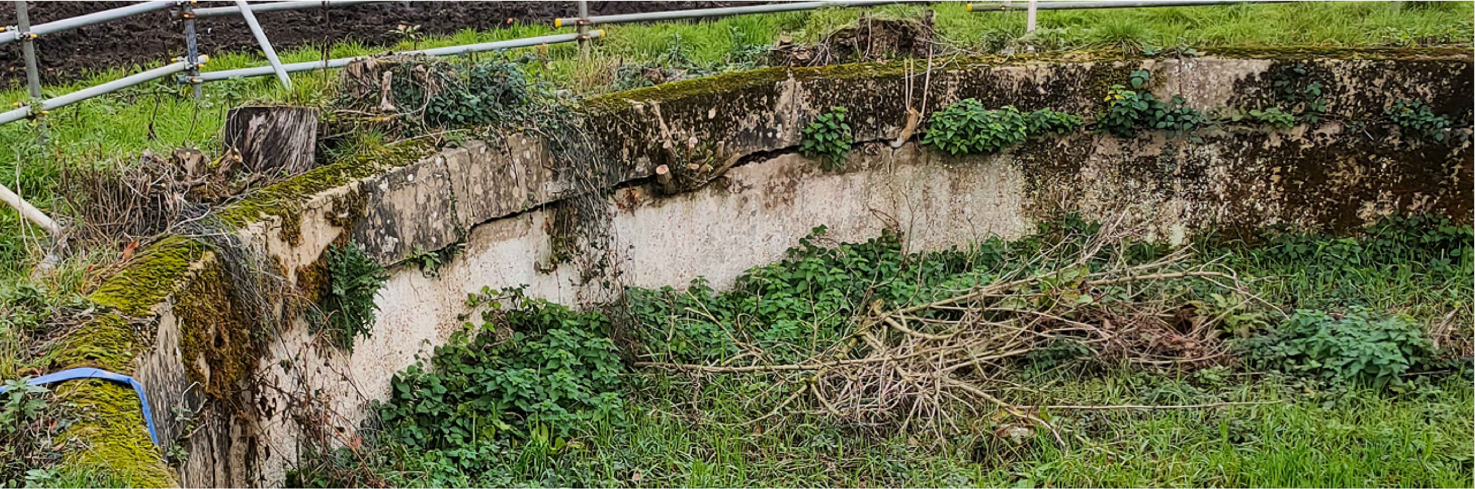
3.State of disrepair of the existing basin perimeter wall
