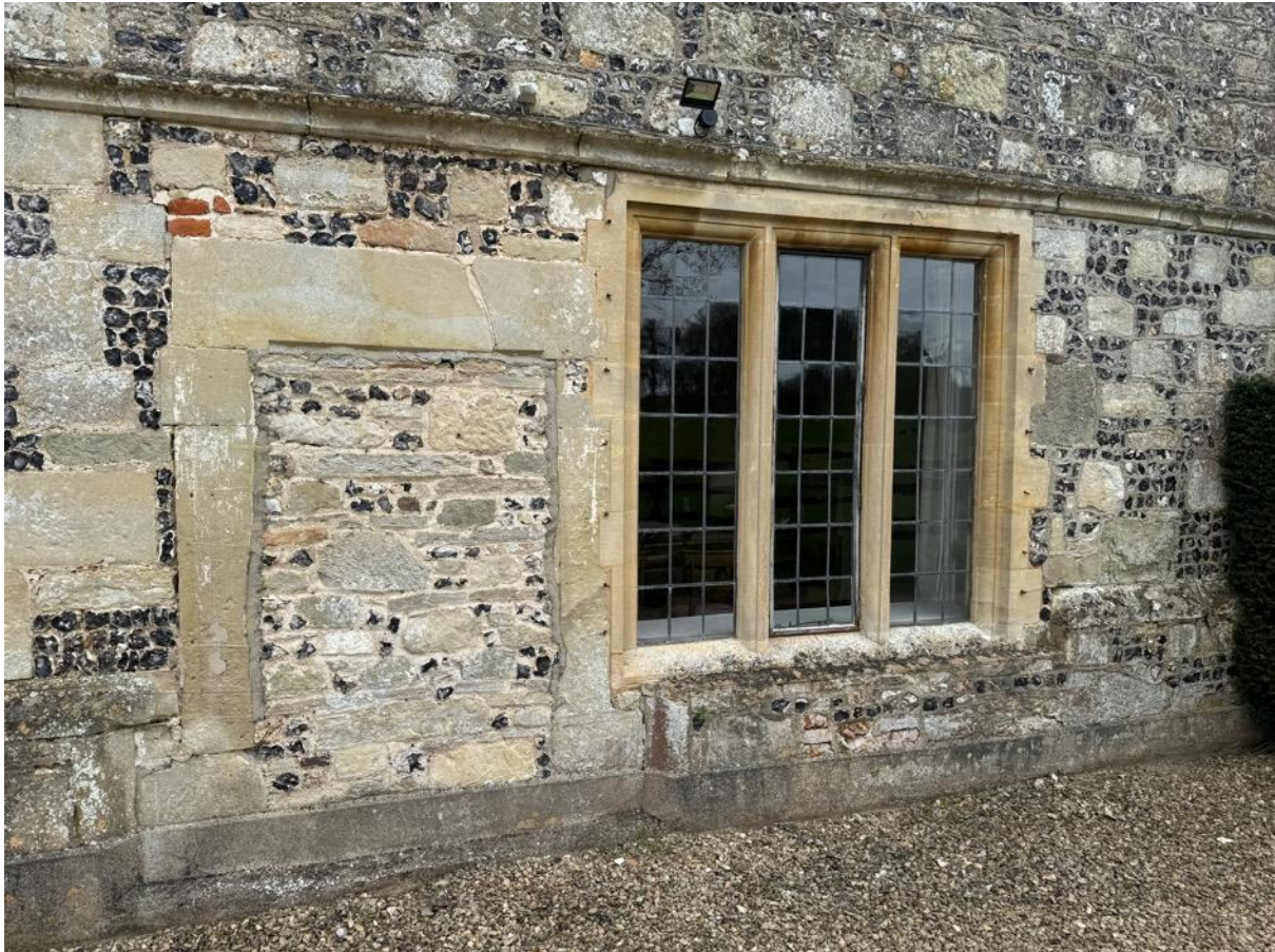
Figure 3: Blocked doorway to billiard room
