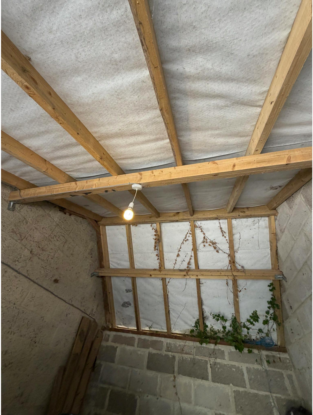
7 - Garage roof showing exposed rafters and Ivy
