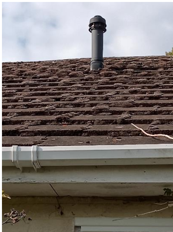
Plate 3. No broken or slipped tiles, rear elevation of B1.
