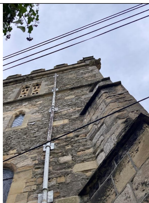
Fig 10. West outlet and down pipe from tower roof. Note: lack of hopper.
