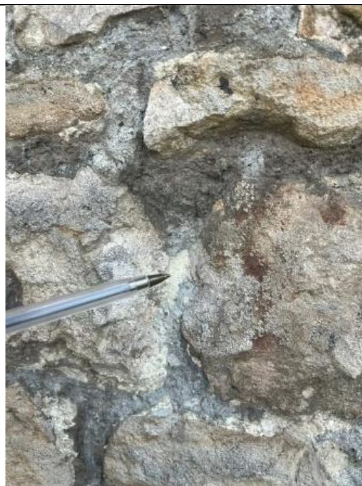
Fig 3. Close up of area of pointing where original pointing mortar is visible beneath the later hard mortar.
