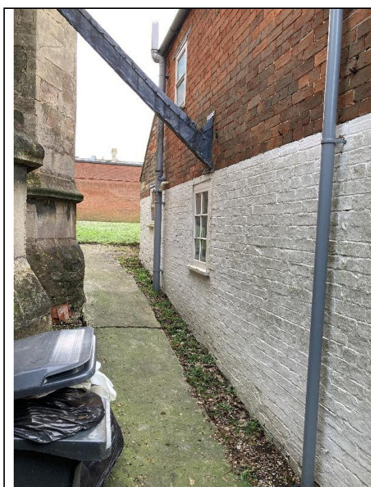
Fig 9. Photo of 'curfew' pipe between Chapel and Cottage which has water ingress into the Cottage.
