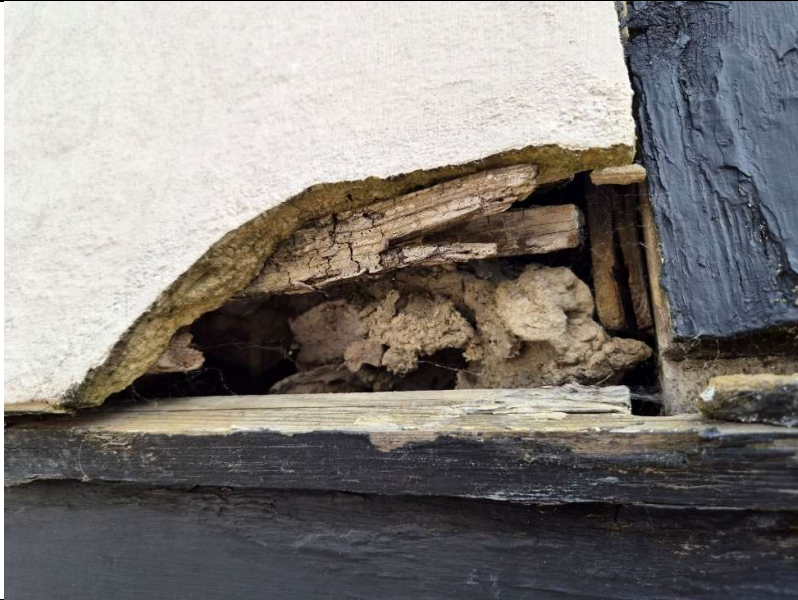
19. Render panel detached from timber laths and at severe risk of falling out. Laths and timber frame now exposed to the elements.
