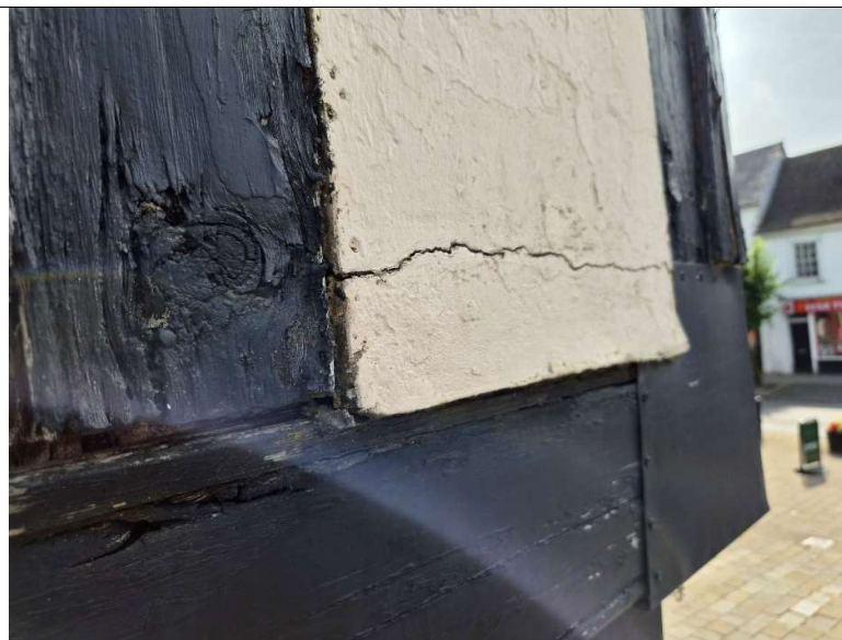
14. Cracked timber and open joints. Note cracked and loose render panel at risk of falling out
