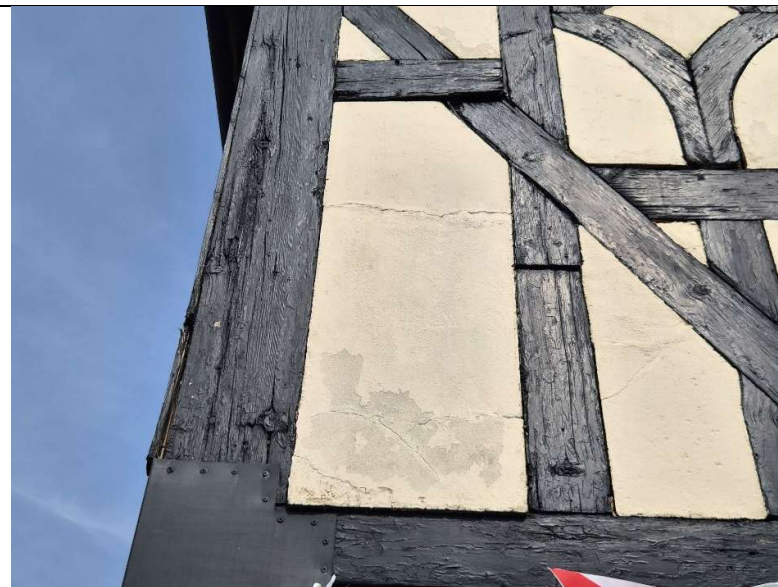
4. Split corner post. Defective render panels and open joints to front (south) corner of building. Note evidence of some historic splice repairs.
