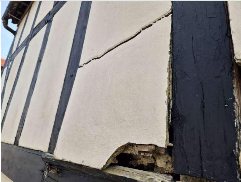
15. Missing section of render to gable end. Note exposed joints to framework
