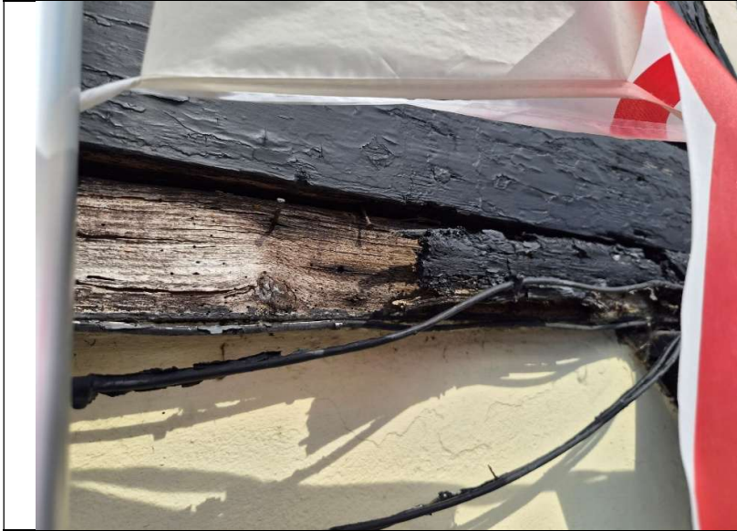
7. Decay noted on bottom member, to left of bay window. Joint indicates some historic repair.
