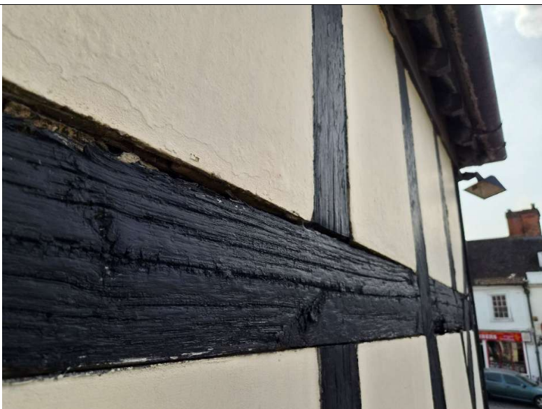
13. Open joints to timber frame and between frame and render panels to gable end.
