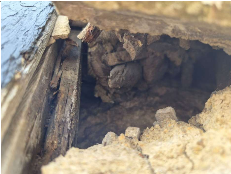
17. Render panel detached from timber laths and at severe risk of falling out. Laths and timber frame now exposed to the elements.
