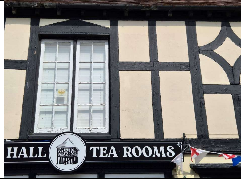
8. View of timber frame and render panels to front elevation. Note cosmetic deterioration to first floor windows.
