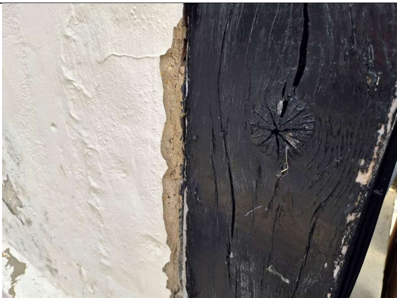
11. Render junction to corner post on southernmost corner of building.
