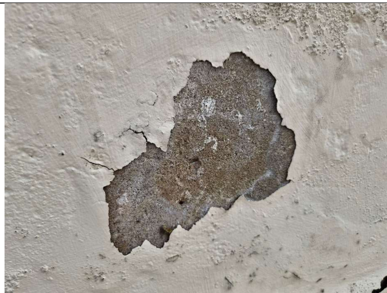
12. Peeling/flaking pant to gable wall, caused by tracking ground moisture
