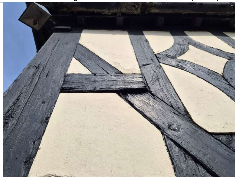
6. Open joints in frame and between timber and render panels – requires repair
