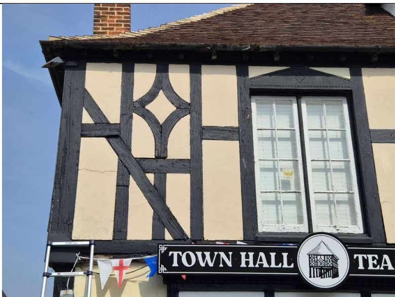
5. View of front part of the building note open joints to frame and cracks to render panels.
