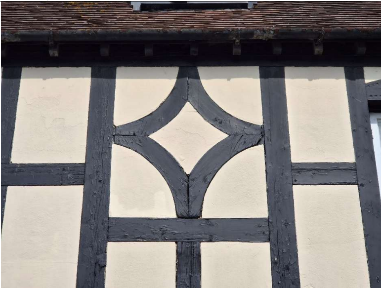
9. Open joints in timber framing to front elevation
