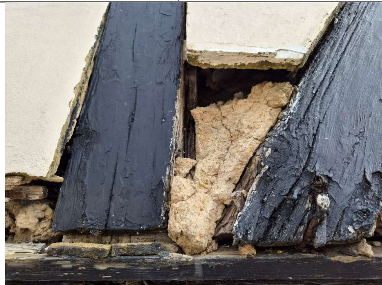
18. Render panel detached from timber laths and at severe risk of falling out. Laths and timber frame now exposed to the elements.
