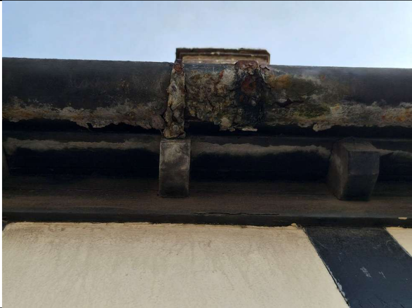
20. Extensive decay of rainwater goods to gable end elevation. Note run-off staining on render panel below, confirming gutter leaks.
