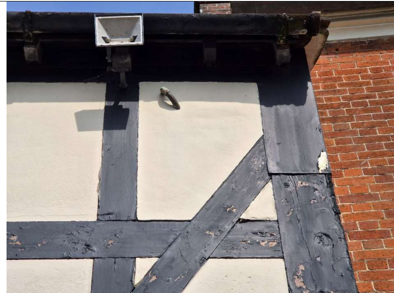
10. Flaking paint and open joints to timber framing. uPVC cover strip to corner post. Open joints around render panels.
