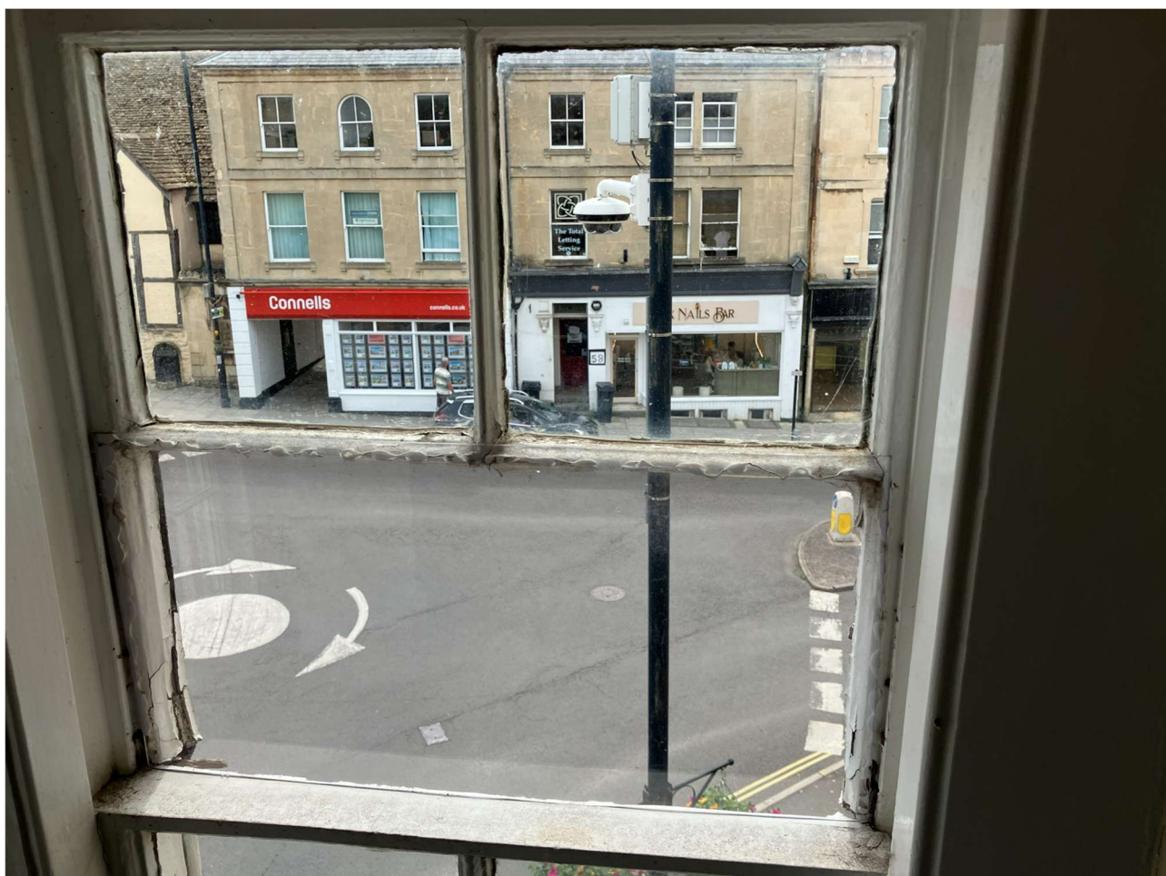
A sash missing a glazing bar and two panes in need of repair
