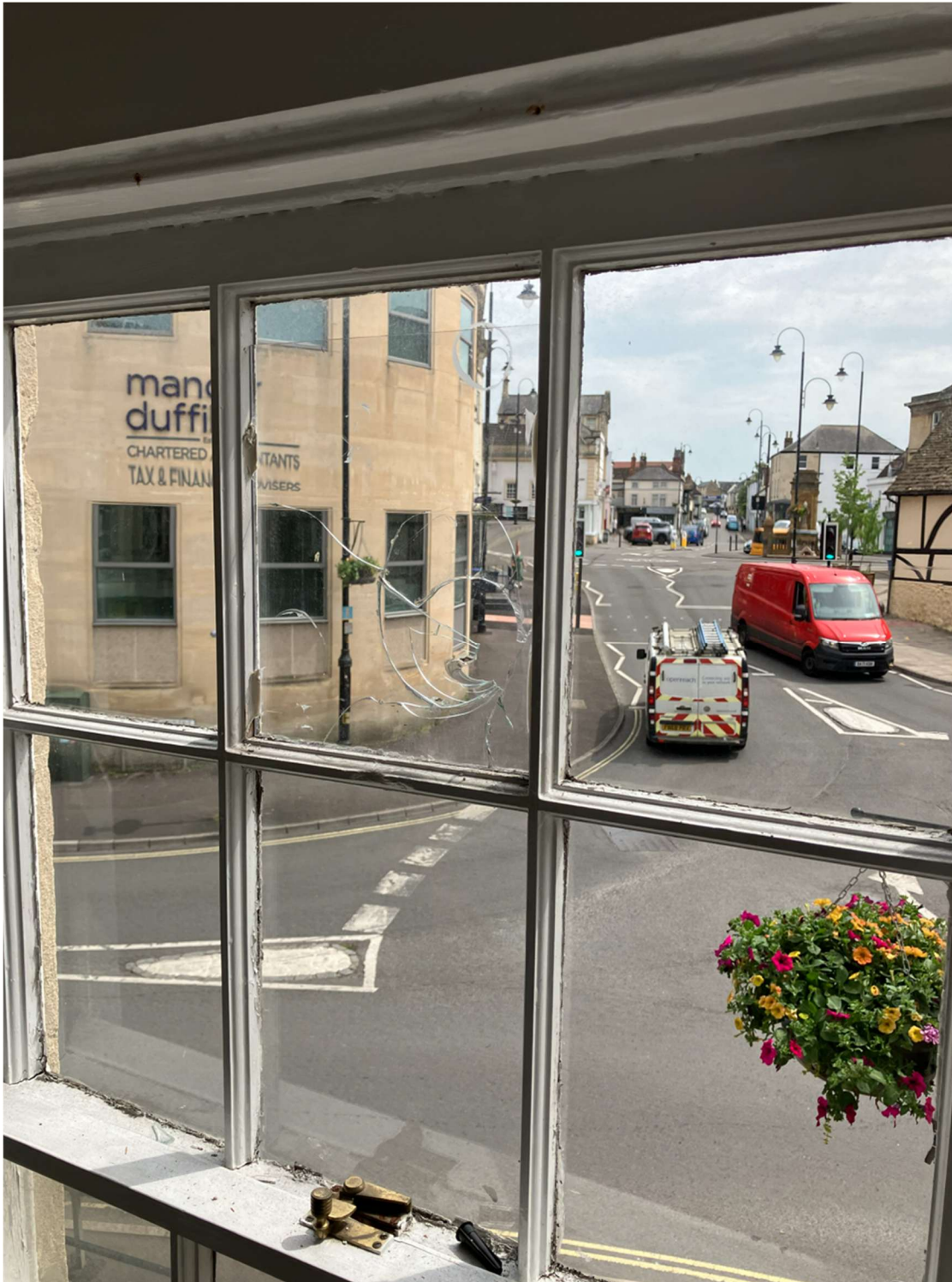
A twentieth century replacement sash with a broken pane
