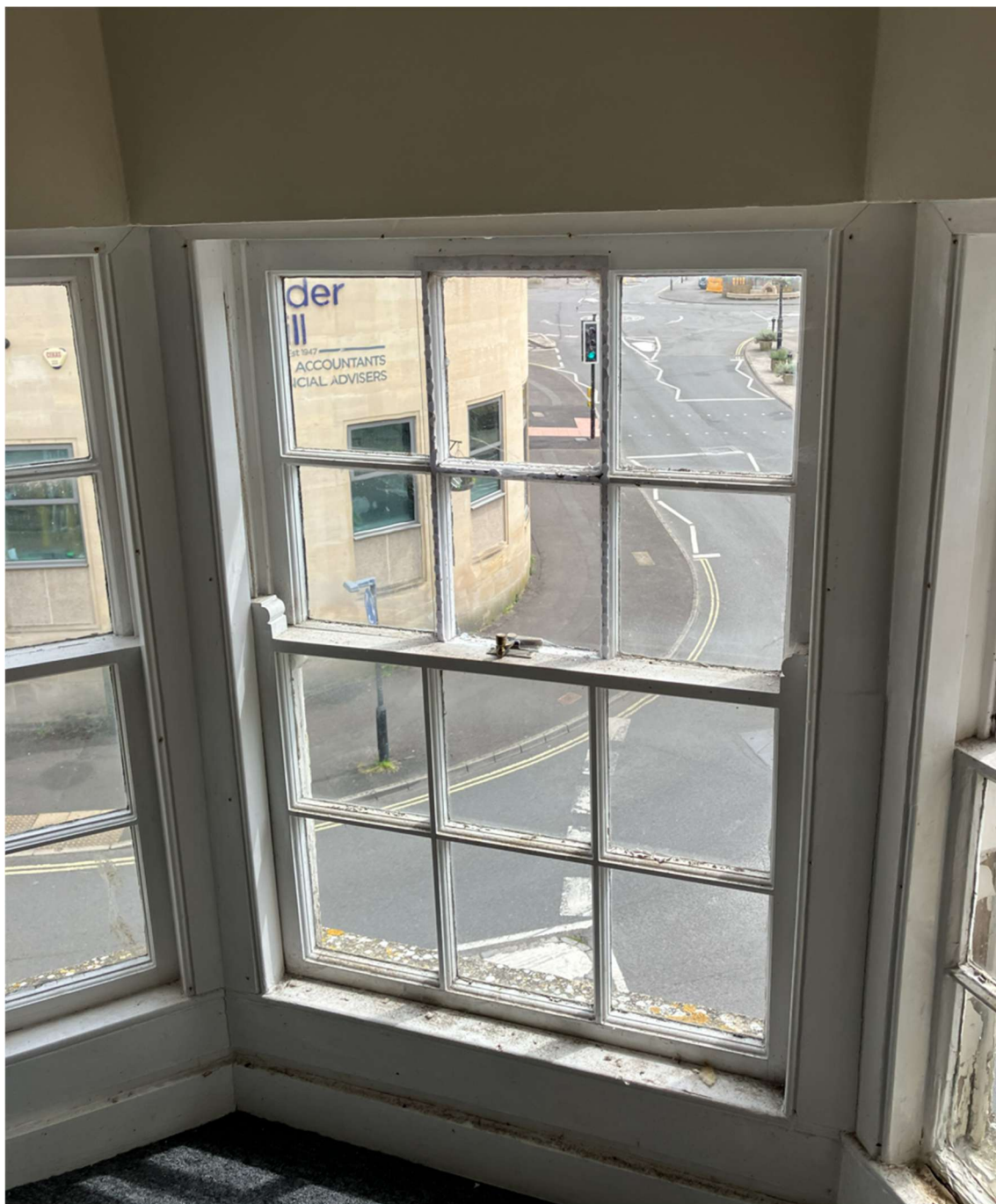
A twentieth-century horned sash window patched up with perspex
