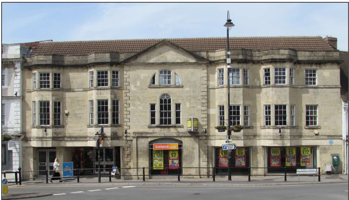
Figure 8: The existing façade of the building with some damaged windows. The roof appears to have been entirely replaced in the 1970s and the Victorian shopfronts replaced by the recessed supermarket windows
