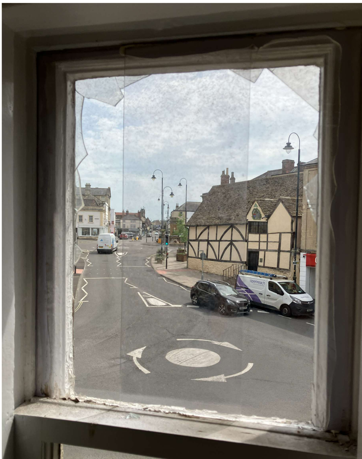
Detail of a broken pane currently patched up with Perspex
