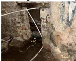
Basement standing water
