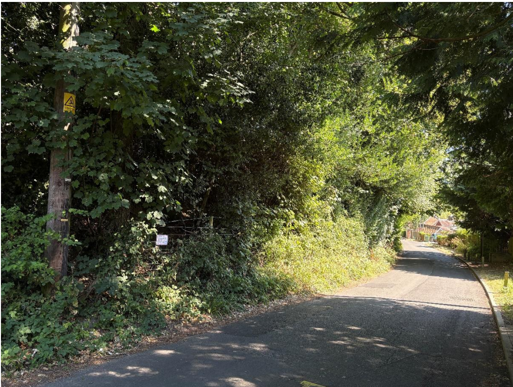
46-1043 Image 5 Vegetation encroachment towards and within the highway.
