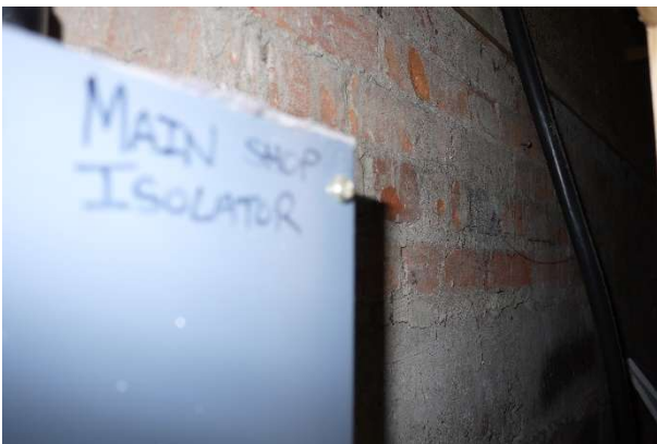
Fig.3 Image of the party wall between 44 and 42 Note the modern brickwork and sand/cement mortar joints. At low level, the wall is covered with a cement slurry.
