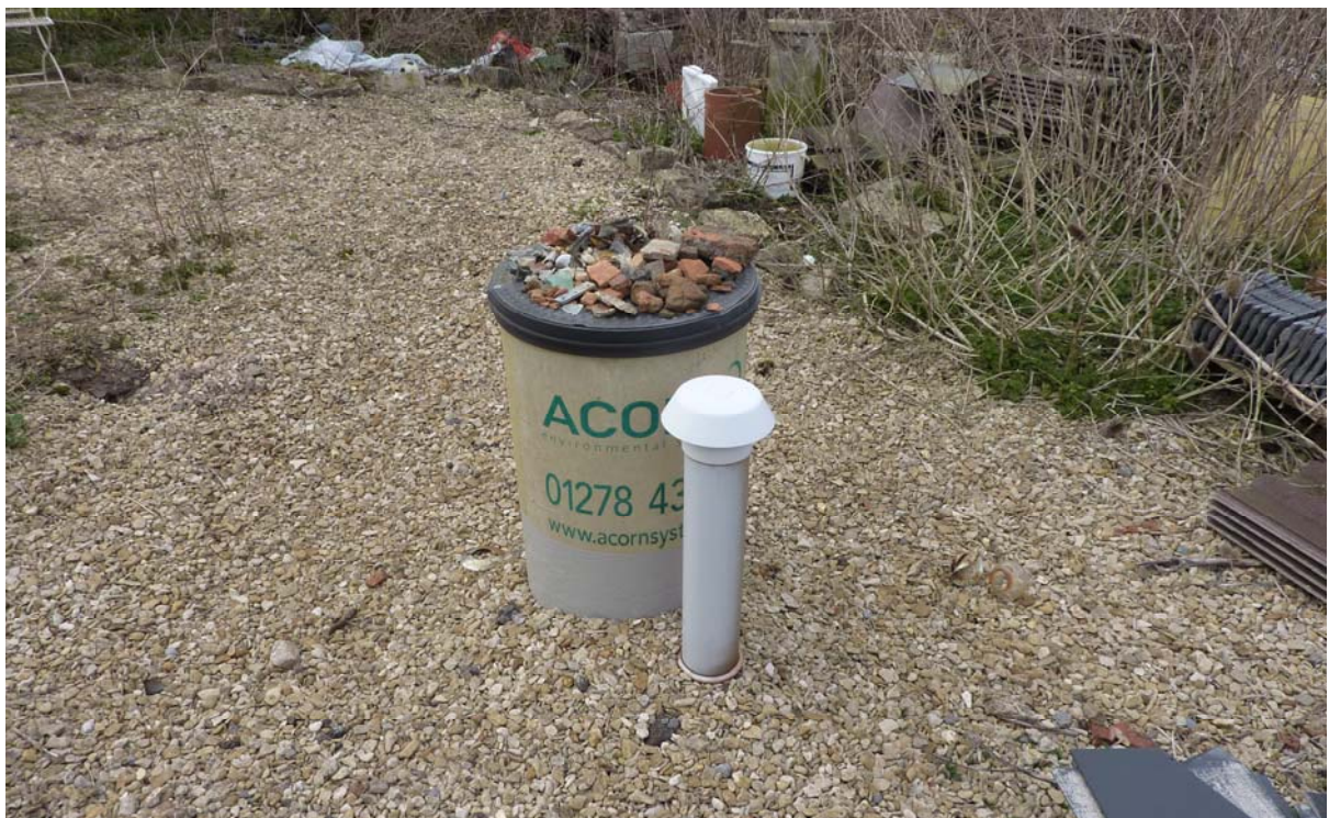
Figure 10: Domestic sewage treatment unit
