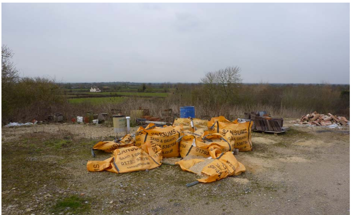
Figure 12: Storage of building materials on northern site area.
