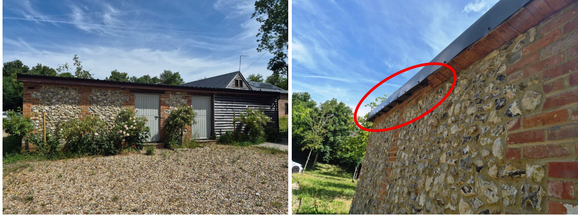
Figure 9 and 10: Southern and western elevations of B2 showing damaged soffit.
