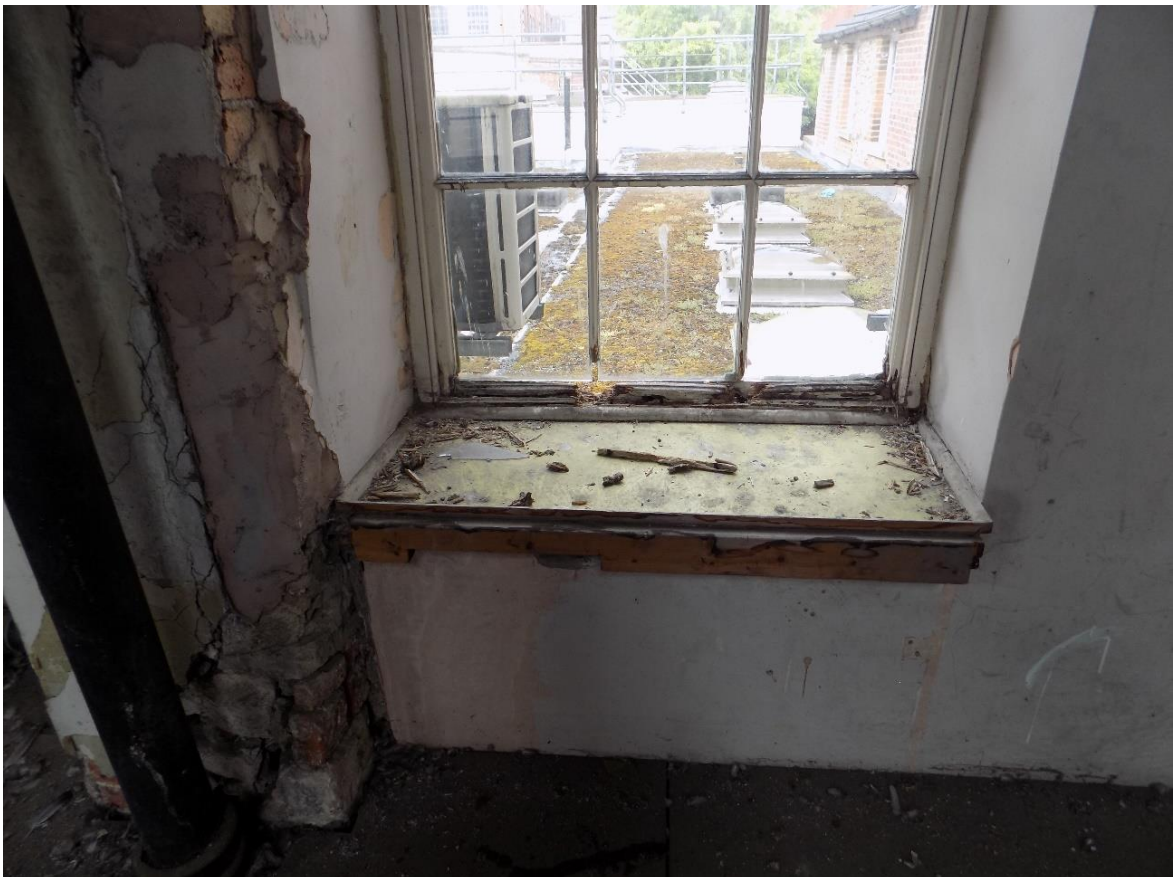
Fig.31: First-floor: Detail of second rear-facing window, showing decayed bottom rail and modern sill.
