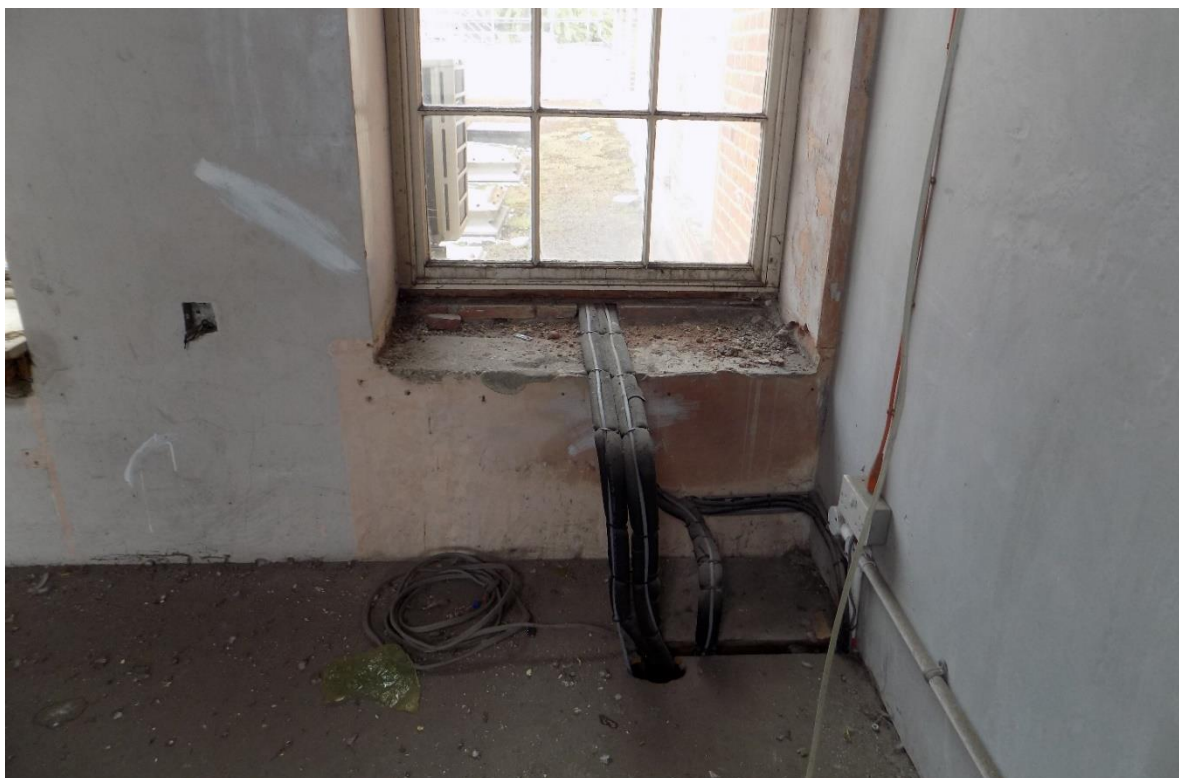
Fig.32: First-floor: Detail of second rear-facing window, showing decayed bottom rail and modern sill.
