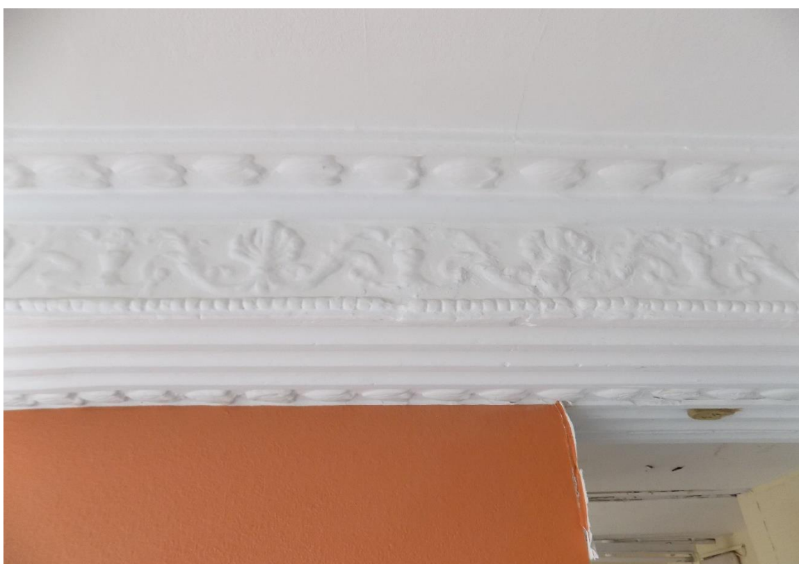
Fig.19: Detail of early eighteenth-century mouldings to beams, showing irregularities.
