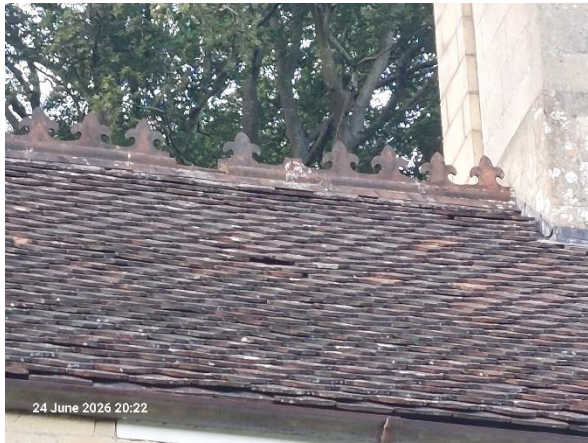
Photo 7: Gaps between the roof tiles.
