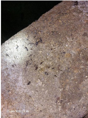
Photo 16: Suspected droppings in the Cellar.
