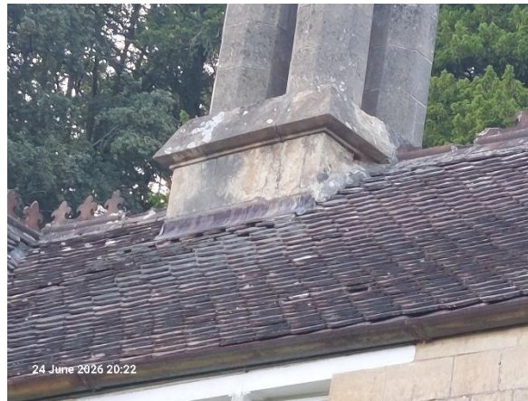
Photo 8: Gaps at the chimney.
