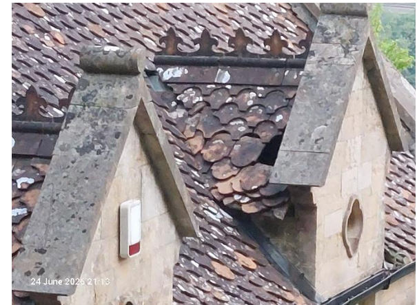
Photo 9: Gap at southernmost dormer window.
