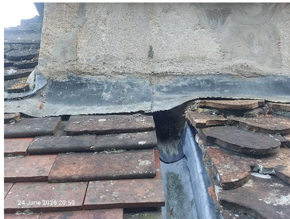
Photo 11: Gaps below chimneys.
