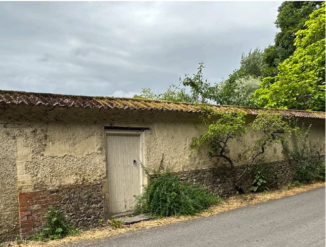
The current cob wall is falling into a state of disrepair. With the removal of the asbestos capping, the wall will need replacing.
