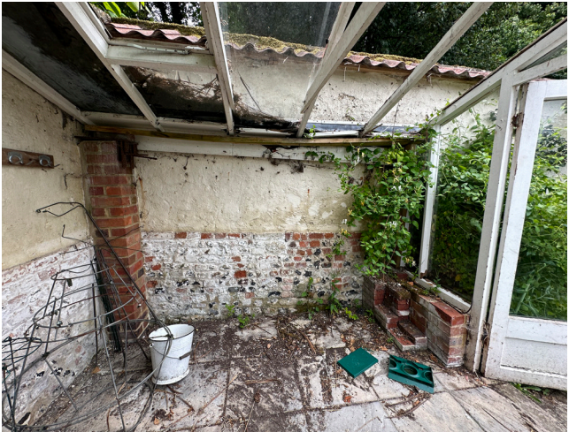
The condition of the greenhouse. Proposal will move the greenhouse to allow the best possible space for the plant room, with the greenhouse suitably re-designed and moved to the end of the plant room.
