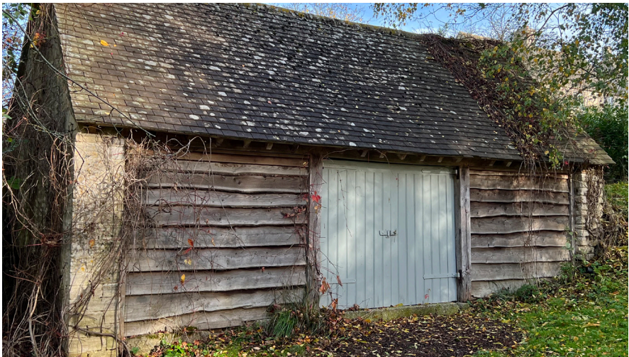
Image: Example of weathered waney edge timber cladding
