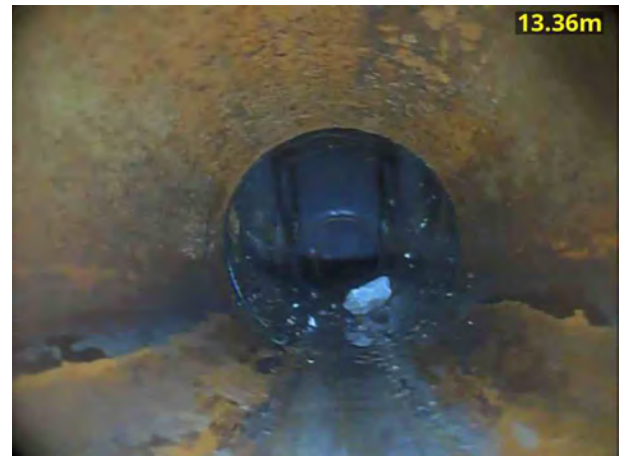
4, 00:01:43, 13.36 m Settled deposits, hard or compacted, 5% cross-sectional area loss, finish, Scale
