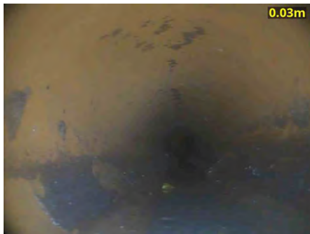
2, 00:00:10, 0.03 m Settled deposits, hard or compacted, 5% cross-sectional area loss, start, Scale
