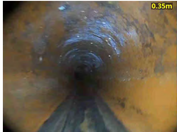
2, 00:00:13, 0.35 m Settled deposits, hard or compacted, 5% cross-sectional area loss, start, Scale
