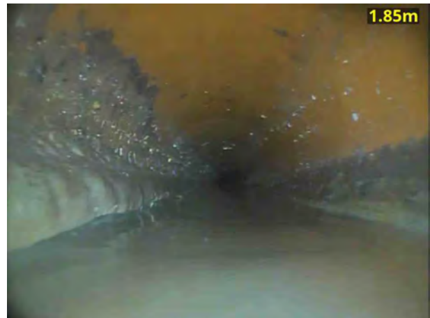
4, 00:00:29, 1.85 m Settled deposits, hard or compacted, 10% cross-sectional area loss
