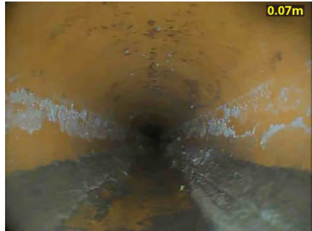
2, 00:00:15, 0.07 m Settled deposits, hard or compacted, 5% cross-sectional area loss, start, Scale
