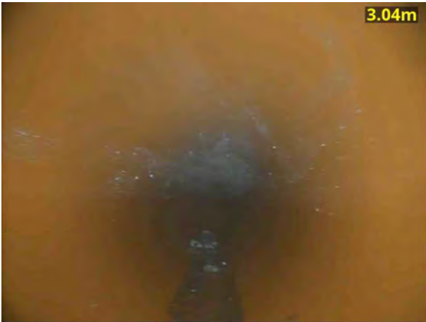
1, 00:07:22, 3.04 m Settled deposits, coarse, 5% cross-sectional area loss
