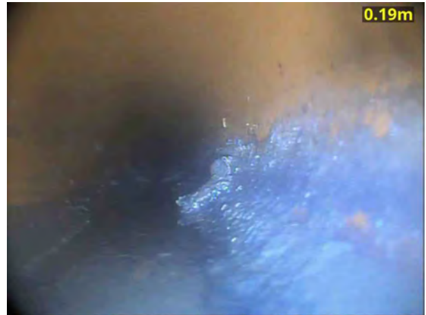
2, 00:00:14, 0.19 m Settled deposits, hard or compacted, 5% cross-sectional area loss, start, Scale
