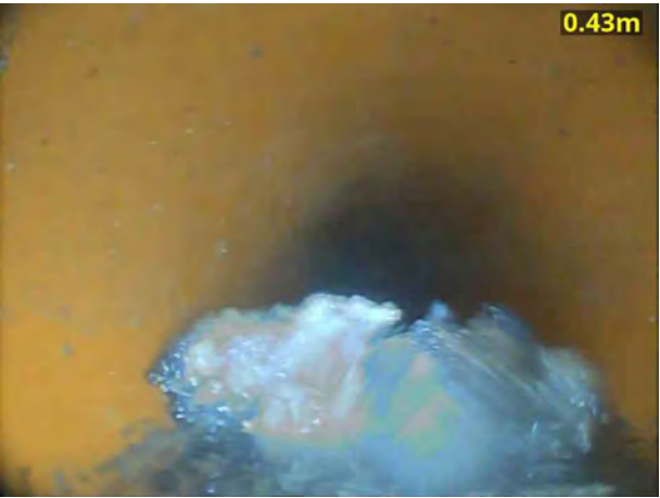
3, 00:00:23, 0.43 m Settled deposits, coarse, 25% cross-sectional area loss
