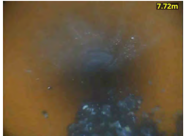
2, 00:06:48, 7.72 m Settled deposits, coarse, 10% cross-sectional area loss
