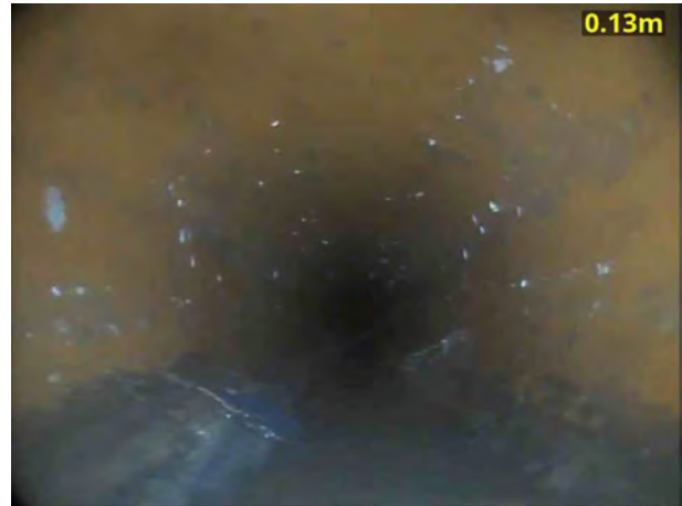
2, 00:00:12, 0.13 m Settled deposits, hard or compacted at joint, 10% cross-sectional area loss, start, Scale
