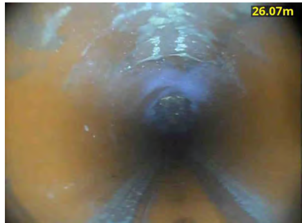
6, 00:02:48, 26.07 m Attached deposits, encrustation at 12 o'clock, 5% cross-sectional area loss, finish
