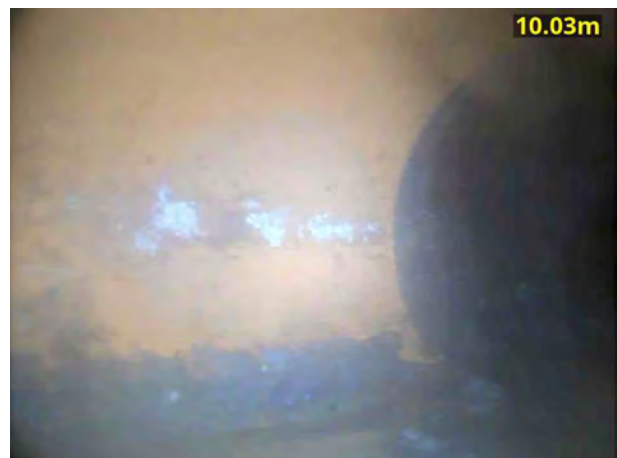
6, 00:01:30, 10.03 m Settled deposits, hard or compacted, 5% cross-sectional area loss, finish, Scale
