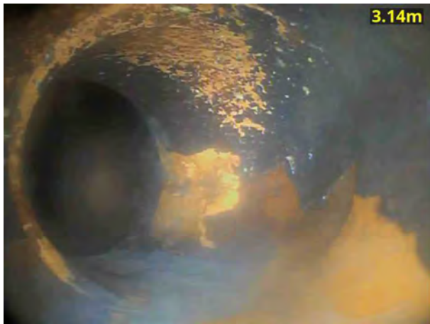
3, 00:00:28, 3.14 m Settled deposits, hard or compacted, 5% cross-sectional area loss, finish, Scale
