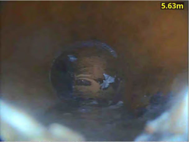
3, 00:00:40, 5.63 m Settled deposits, hard or compacted, 5% cross-sectional area loss, finish
