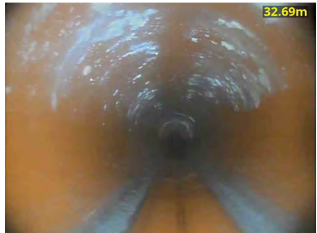
10, 00:03:27, 32.69 m Attached deposits, encrustation from 10 o'clock to 2 o'clock, 5% cross-sectional area loss, finish
