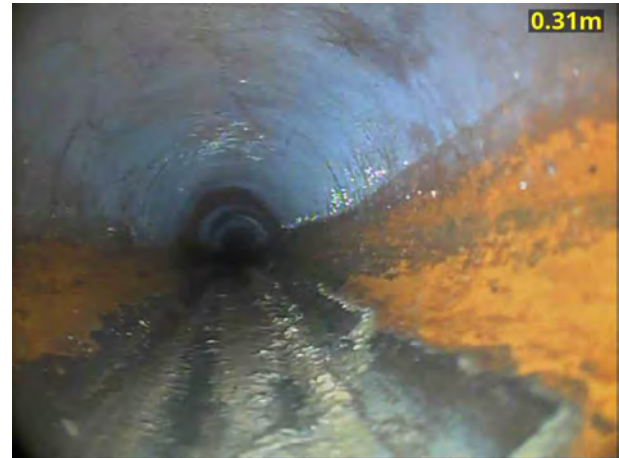
2, 00:00:14, 0.31 m Settled deposits, hard or compacted, 5% cross-sectional area loss, start, Scale
