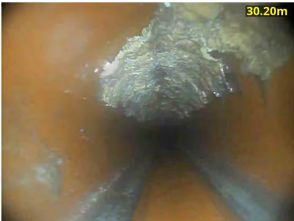
9, 00:03:12, 30.20 m Attached deposits, encrustation from 10 o'clock to 2 o'clock, 5% cross-sectional area loss, start
