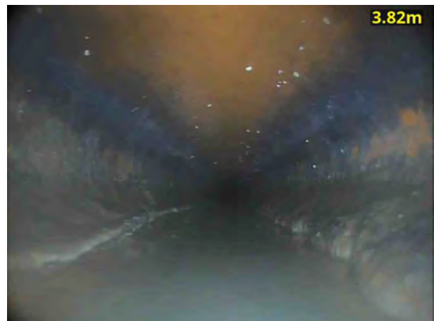
4, 00:00:39, 3.82 m Settled deposits, hard or compacted, 15% cross-sectional area loss
