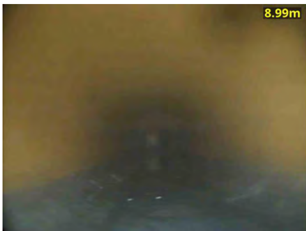
5, 00:01:20, 8.99 m Settled deposits, hard or compacted, 5% cross-sectional area loss, start, Scale
