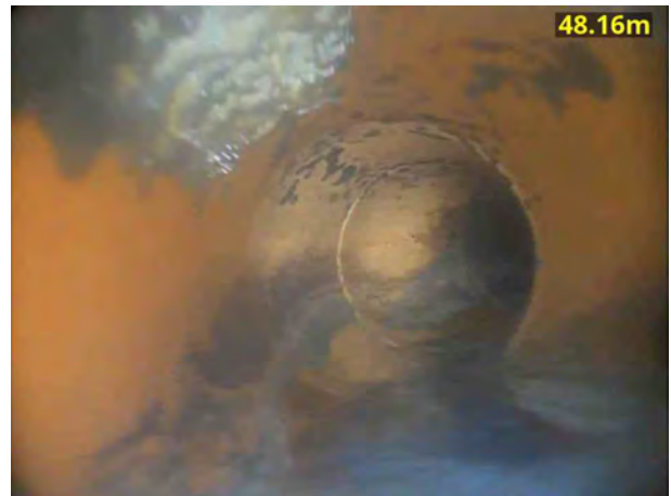
12, 00:04:50, 48.16 m Attached deposits, encrustation from 9 o'clock to 3 o'clock, 5% cross-sectional area loss, finish
