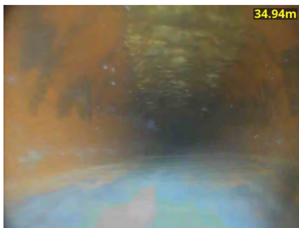
6, 00:04:05, 34.94 m Attached deposits, grease from 10 o'clock to 2 o'clock, 10% cross-sectional area loss, start
