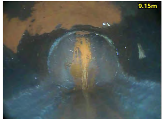
4, 00:00:16, 9.15 m Settled deposits, hard or compacted, 10% cross-sectional area loss, finish, Scale
