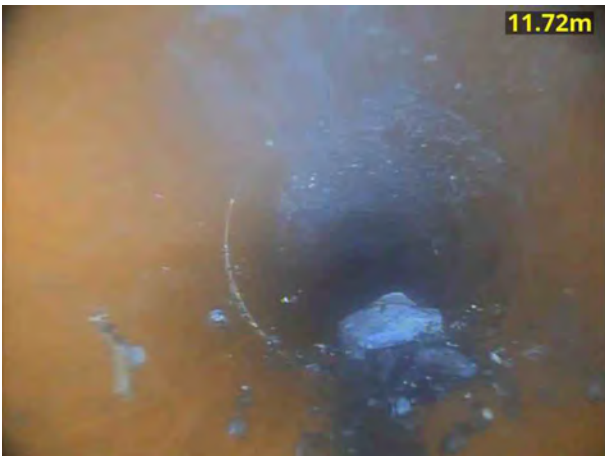
3, 00:06:17, 11.72 m Settled deposits, other, 5% cross-sectional area loss, Grease/fat
