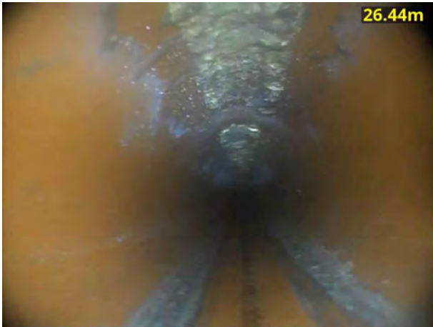
7, 00:02:50, 26.44 m Attached deposits, encrustation at 12 o'clock, 5% cross-sectional area loss, start
