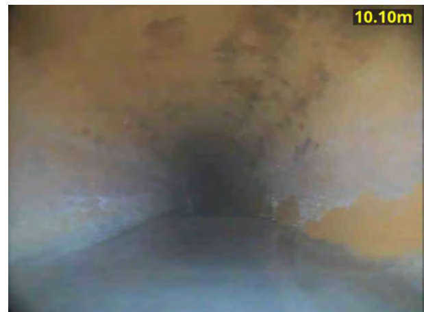
4, 00:01:17, 10.10 m Settled deposits, hard or compacted, 5% cross-sectional area loss, finish
