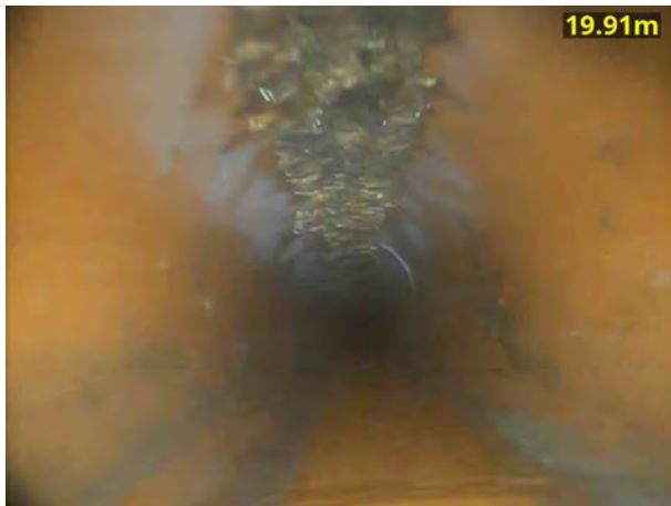
5, 00:02:12, 19.91 m Attached deposits, encrustation at 12 o'clock, 5% cross-sectional area loss, start
