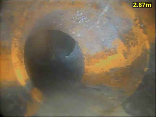
3, 00:00:28, 2.87 m Settled deposits, hard or compacted, 5% cross-sectional area loss, finish
