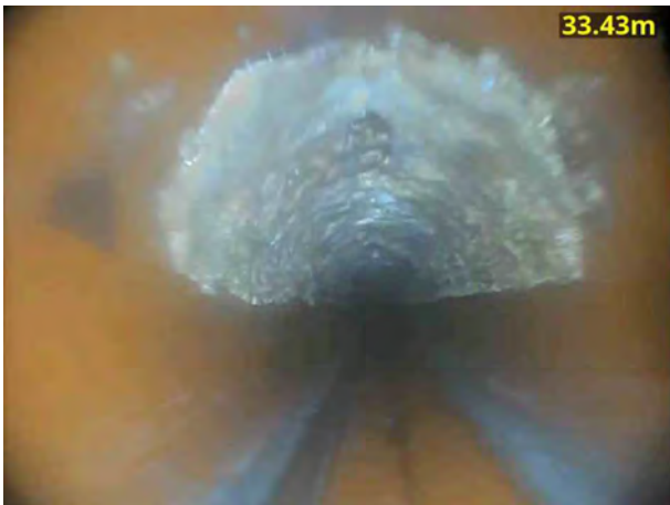
11, 00:03:31, 33.43 m Attached deposits, encrustation from 9 o'clock to 3 o'clock, 5% cross-sectional area loss, start
