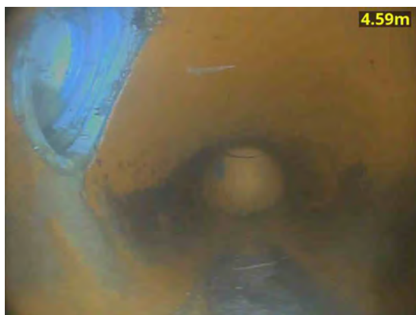
4, 00:00:43, 4.59 m Connection other than junction at 10 o'clock, 40mm dia
