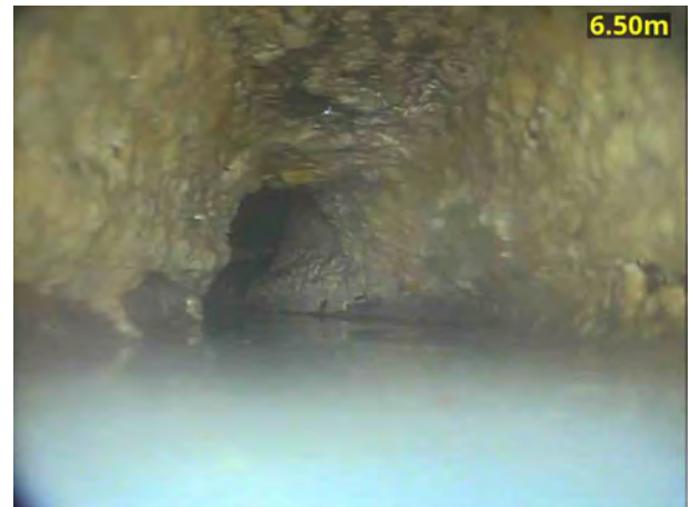
4, 00:01:12, 6.50 m Attached deposits, encrustation from 9 o'clock to 3 o'clock, 25% cross-sectional area loss, finish
