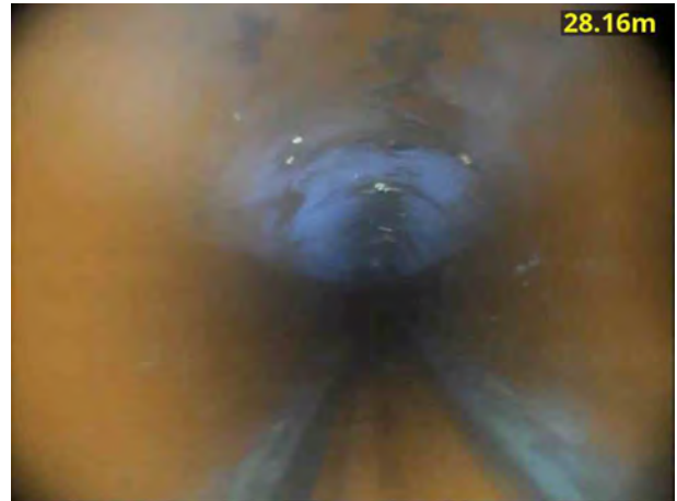
8, 00:03:00, 28.16 m Attached deposits, encrustation at 12 o'clock, 5% cross-sectional area loss, finish
