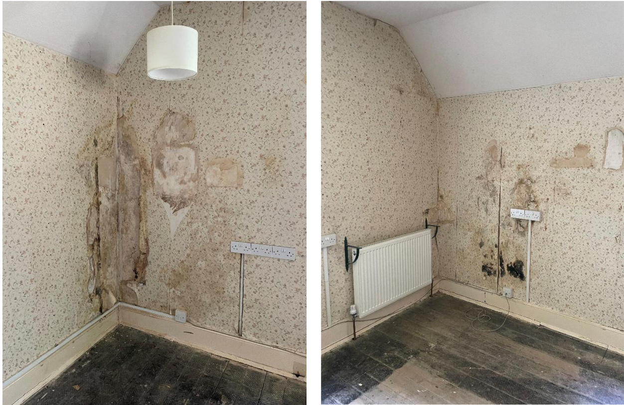
Figures 25 and 26 – There is serious water ingress at 1 st floor level in Bedroom 1 primarily due to the poor condition of the roof.
