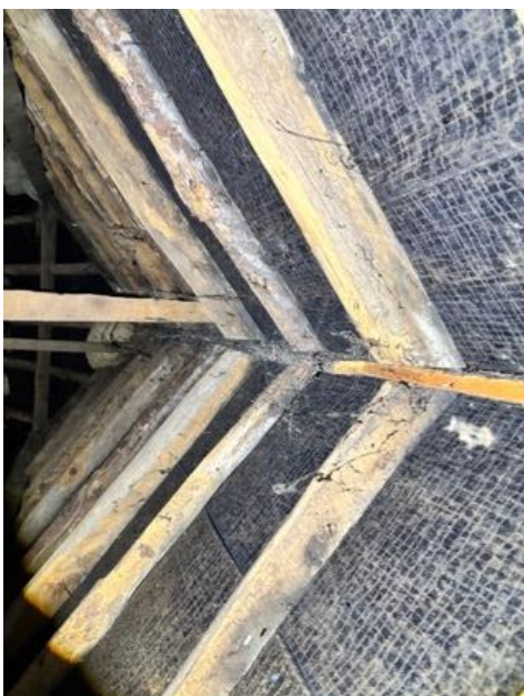
Ridge board heavily cobwebbed within main loft at The Silver Plough
