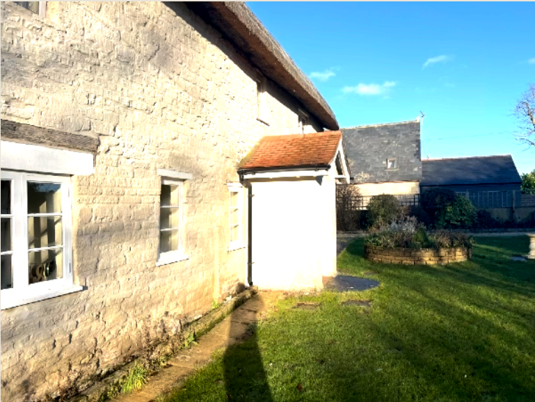
Figure 5– Existing 1973 front porch. Patch of brickwork repair to base of chalk stone wall of cottage
